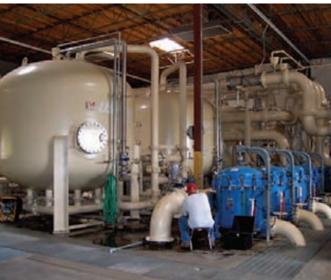
Left: Groundwater treatment facility at Aerojet Superfund site.
