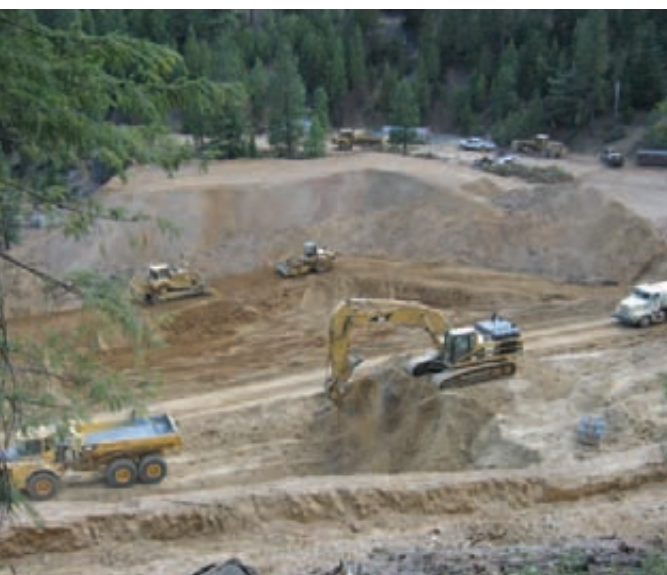
Left: Heavy equipment prepares disposal site for mercury-contaminated mining waste removed from creekbed.
