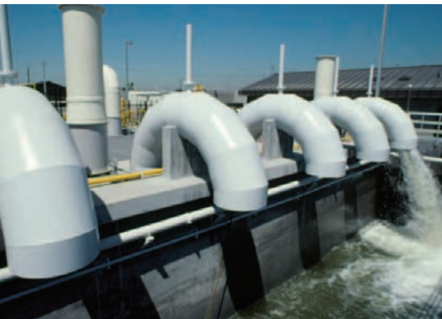
The Oakport Wet Weather Facility processes excess sewage diverted from EBMUD's wastewater collection system.
