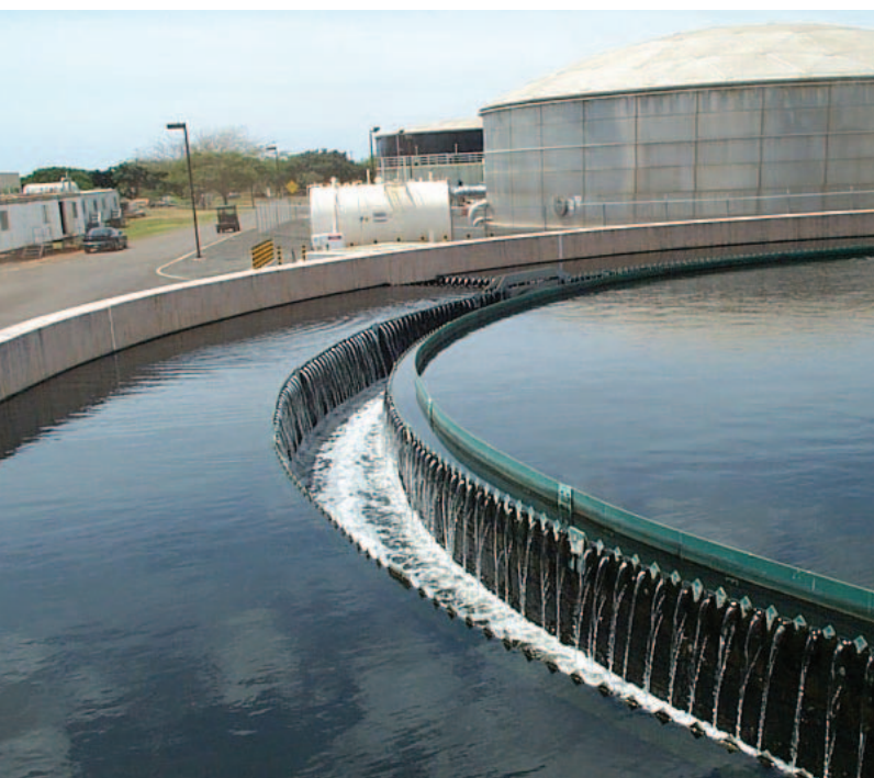
A clarifier at the Honouliuli treatment facility in Honolulu.
