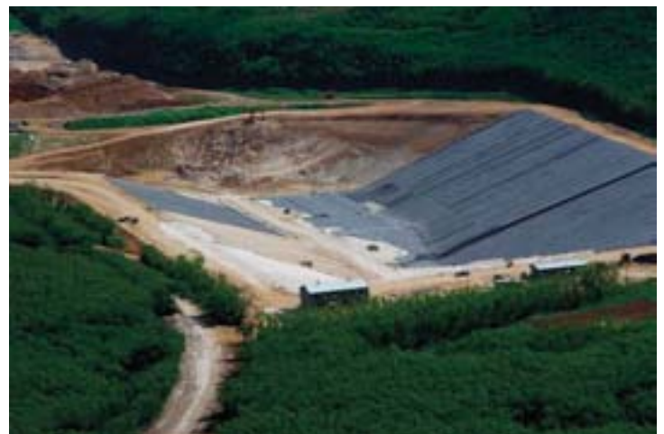
Saipan's new Marpi Landfill under construction. The new solid waste landfill, first in the Pacific Islands to comply with federal standards for preventing pollution, opened in February 2003.
