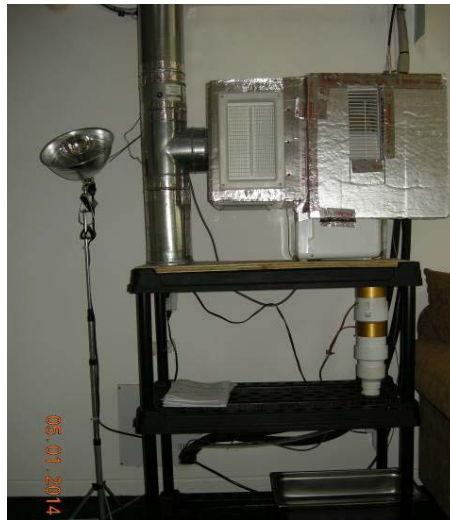
Figure 4. Stand-alone dehumidifier with OA intake plenum constructed on the left side
