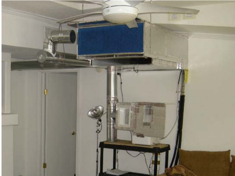
Figure 5. MSHP indoor unit mounted high on the wall in the MH Lab main space. The return air of the unit is enclosed in a plenum with a calibrated flow station. As shown, the OA duct terminates at the intake to the MSHP. It can also be directed to the dehumidifier unit below the MSHP or redirected further into the central space.
