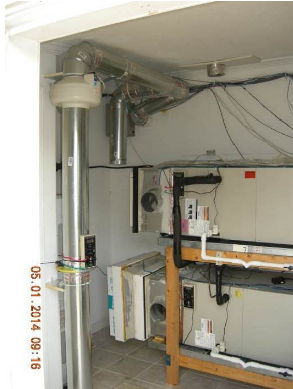
Figure 3. Mechanical ventilation OA is brought into the MH Lab using an in-line fan and measured with a calibrated iris damper. This photo shows the option that delivers the air near the return of the SEER 22 (top) and SEER 13 central systems.
