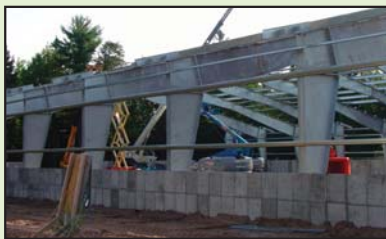
Above: Construction projects, like the one at Pendills Creek National Fish Hatchery pictured here, boost the Service's capacity to rear trout while concurrently benefiting local economies through the use of local contractors. Service photo.
