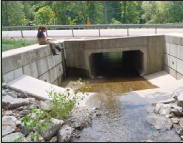
Above: Road-crossing over Honeoye Creek; identified by field assessment to block fish passage. Service photo by Ray Li.
