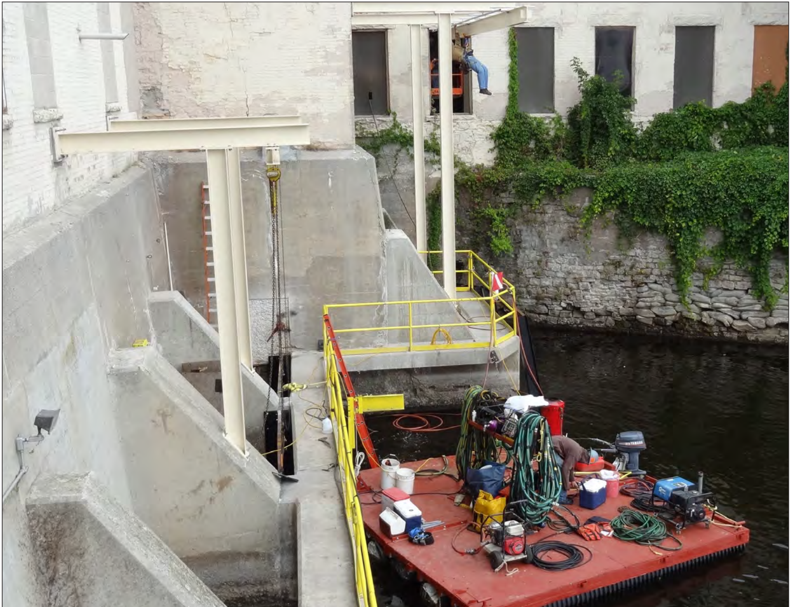
Divers inspect the river bottom as workers install a de-watering system that will allow access and construction of a fishway for lake sturgeon at a hydropower dam located on the Menominee River in northern Wisconsin. Rory Alsberg, North American Hydro.
