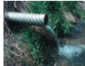
Figure 3. Tile outlet into drainage ditch
