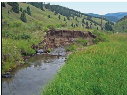
Figure 2. A cut bank on Comanche Creek, before treatment.
