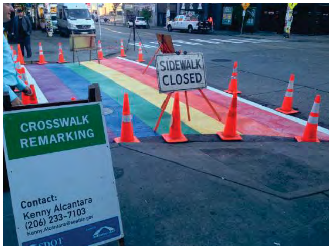
Figure 6: Rainbow crosswalk being installed, Capitol Hill neighborhood, Tenth Avenue and East Pike Street, Seattle, Washington, 2015. Photo by Gordon Werner. 58
