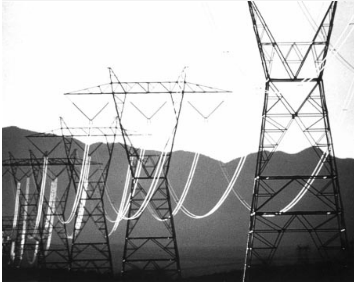
High-tension power lines and towers. Source: U.S. Department of Energy.
