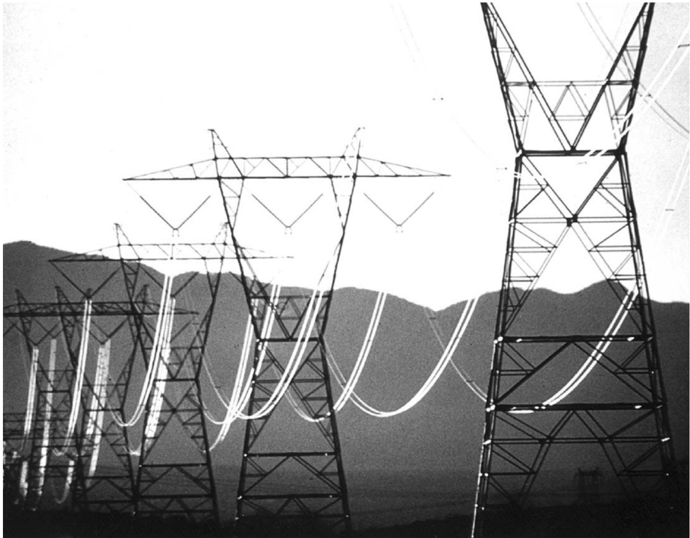
High-tension power lines and towers. Source: U.S. Department of Energy.
