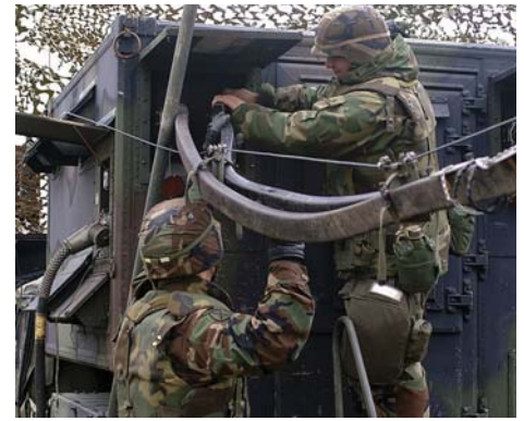
Soldiers from the 5th Signal Command hook up cables to the communications shelter from a tropospheric scatter radio antenna.
