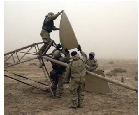
Soldiers from the 11th and 93rd Signal Brigades set up a tropospheric scatter antenna during a sandstorm during the first days of hostilities in Iraq.
