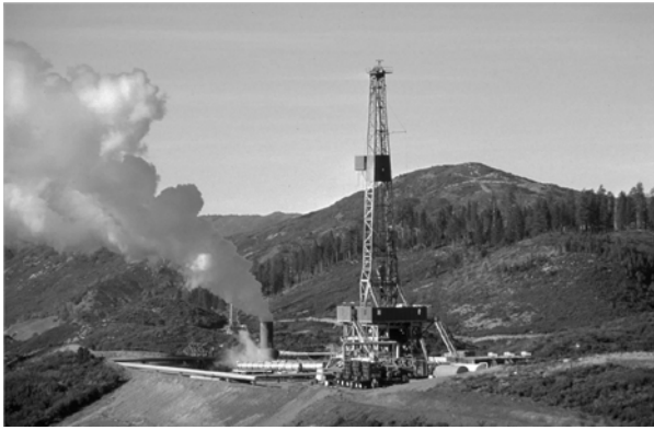
Figure 1: Rig at The Geysers geothermal field in in Middletown, California. This EGS demonstration project, funded by DOE and cost-shared with industry, has shown the potential to produce 5 megawatts from an engineered reservoir in a deep, impermeable, and unproductive rock body, with far greater additional potential at this site. (Photo credit: Calpine; Geothermal Technologies Program 2012 Peer Review)
