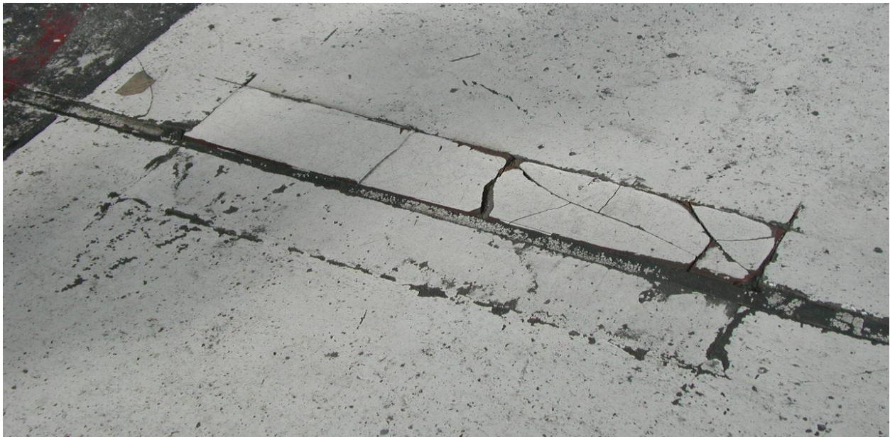
Figure 9. Typical example of minor spalling in concrete floor slab (Mr. Richard Simonton, 2013).
