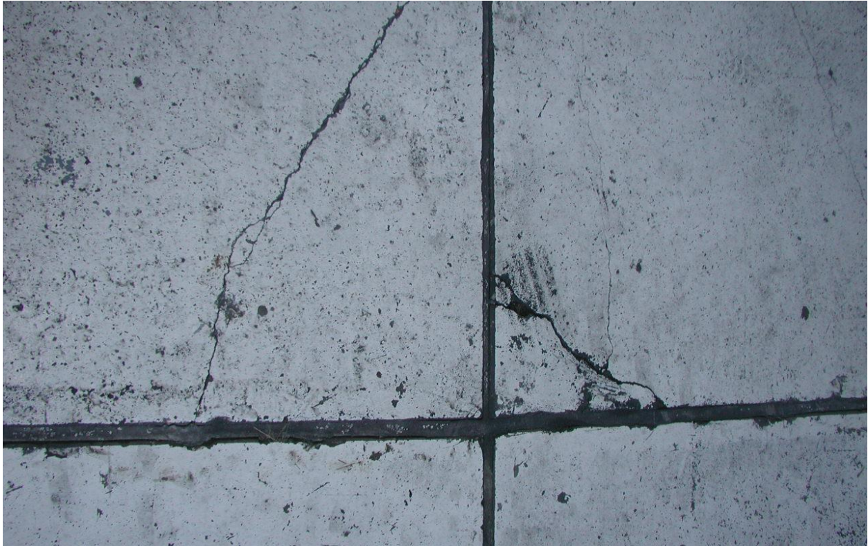
Figure 8. Typical example of minor cracking in concrete floor slab (Mr. Richard Simonton, 2013).
