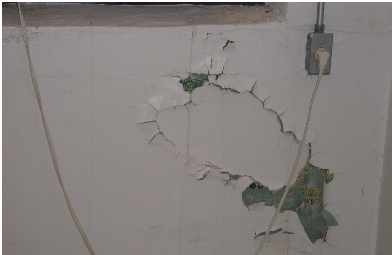
Figure 15. Example of moisture problems on interior face of exterior wall (Mr. Richard Simonton, 2013).
