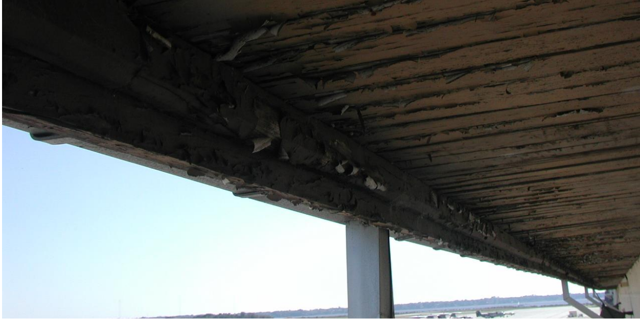
Figure 13. Severe paint peeling at wood tongue-and-groove soffit on north side of Hangar 113 (Mr. Richard Simonton, 2013).
