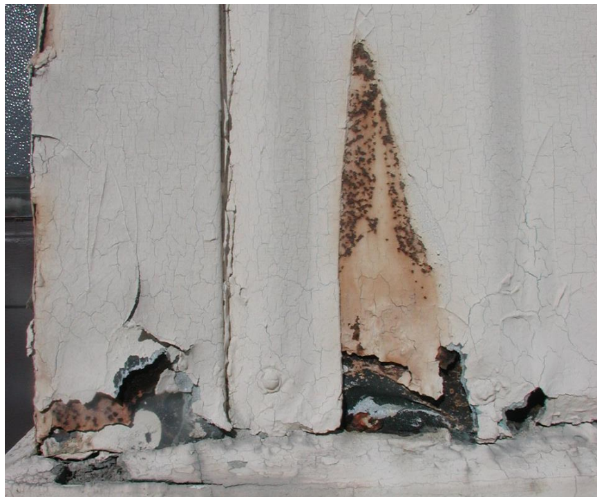
Figure 21. Typical deterioration of corrugated wall panels where bottom of panels abut concrete knee walls (Mr. Richard Simonton, 2013).
