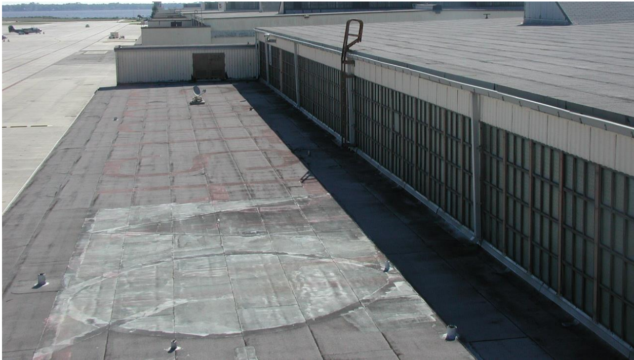
Figure 12. Existing modified bitumen roof near end of service life on Hangar 113 (Mr. Richard Simonton, 2013).
