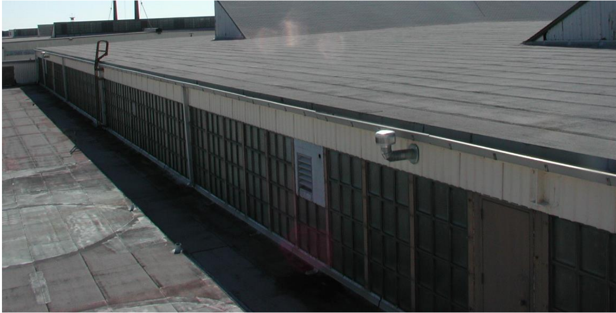
Figure 17. Typical example of original clerestory windows remaining north and south sides of hangar (Mr. Richard Simonton, 2013).
