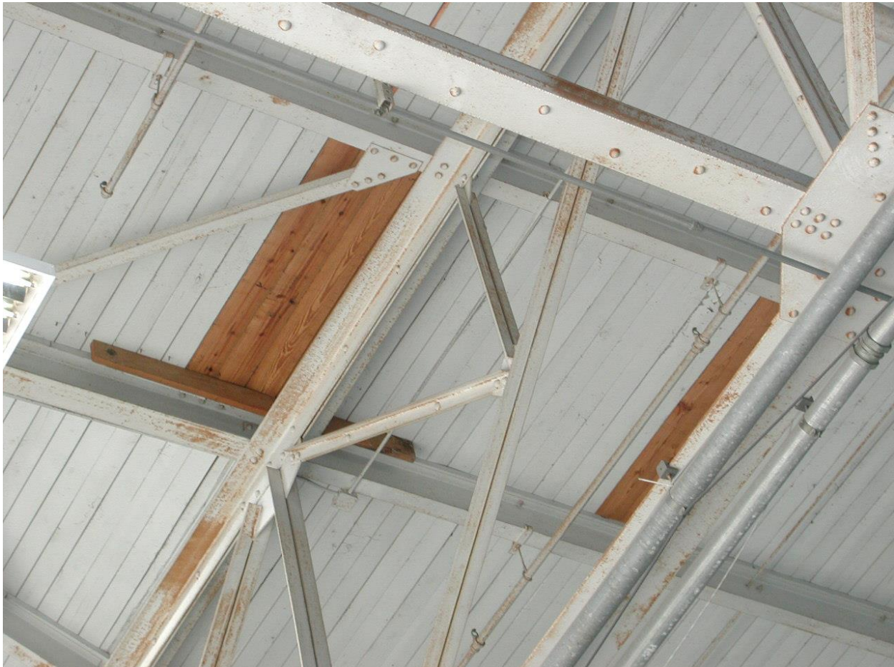
Figure 10. Typical example of spotted corrosion and wood roof deck replacement on Hangar 113 (Mr. Richard Simonton, 2013).
