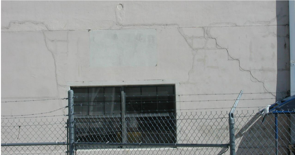
Figure 16. Example of exterior cracks in stucco and concrete masonry units at south elevation of Hangar 113 (Mr. Richard Simonton, 2013).
