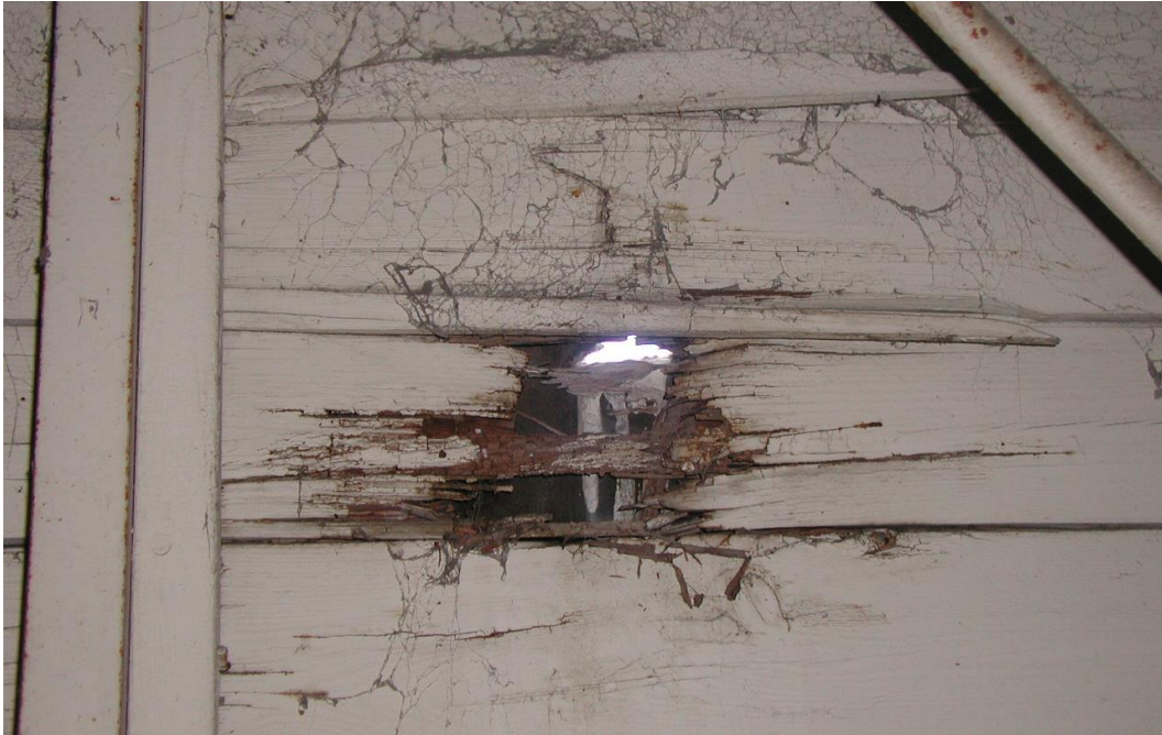
Figure 20. Example of damage to tongue-and-groove wood plank substrate in hangar door pockets and spotted corrosion on steel framing (at upper right) (Mr. Richard Simonton, 2013).
