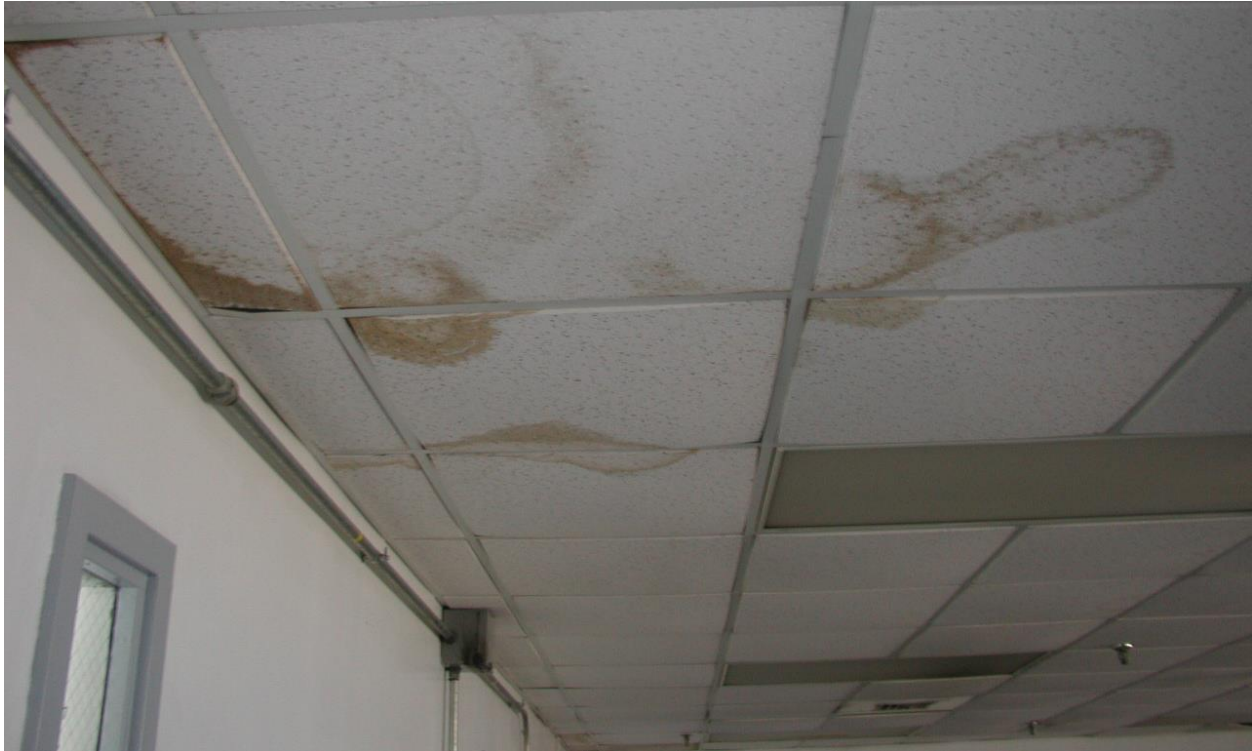
Figure 30. Suspended ceiling with water damage (Mr. Richard Simonton, 2013).
