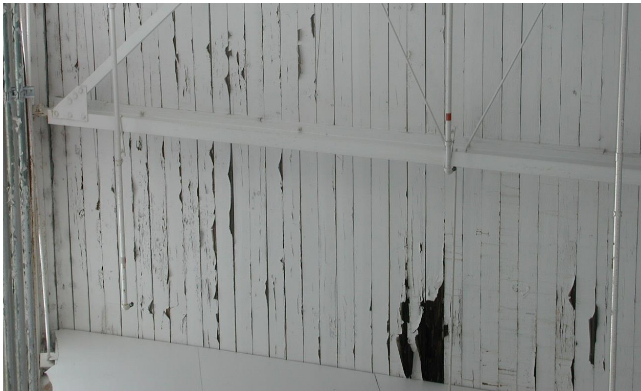
Figure 11. Peeling paint indicating possible moisture damage at wood deck above sawtooth clerestory (Mr. Richard Simonton, 2013).
