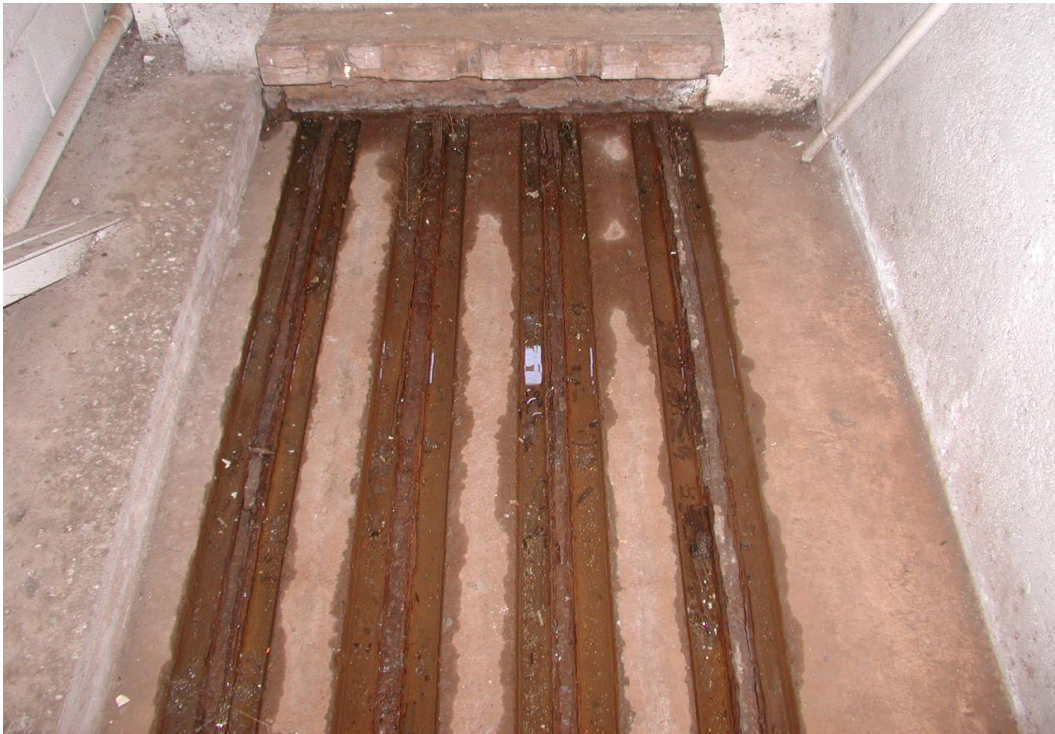
Figure 27. Interior view of hangar door pocket showing steel rails with severe section loss and standing water in concrete recess (Mr. Richard Simonton, 2013).
