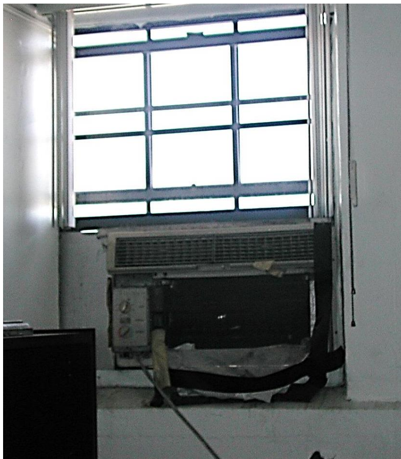
Figure 32. Example of window air-conditioning unit for offices (Mr. Richard Simonton, 2013).
