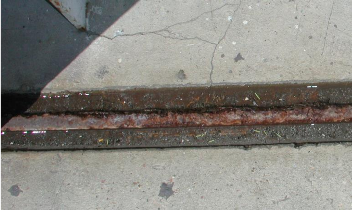
Figure 26. View of hangar door rail with reduced steel section (Mr. Richard Simonton, 2013).
