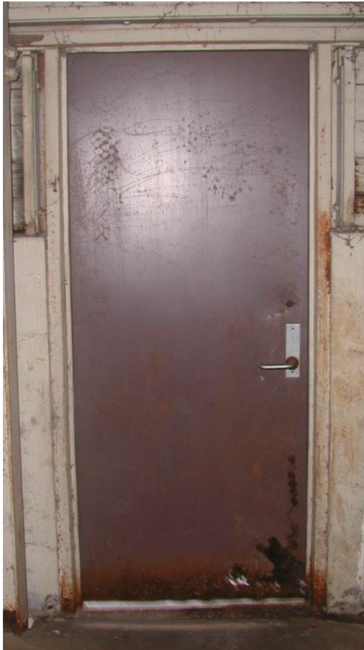
Figure 22. Typical exterior man door that needs replacement (Mr. Richard Simonton, 2013).
