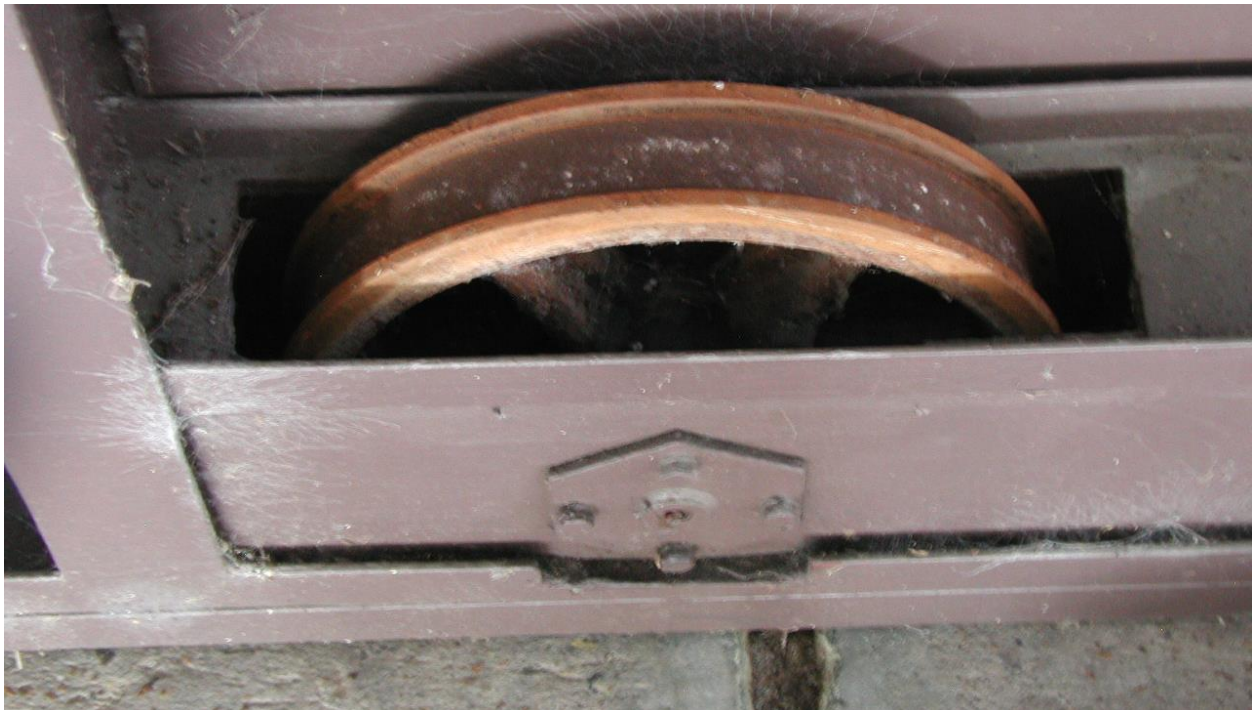
Figure 25. Typical hangar door roller (Mr. Richard Simonton, 2013).
