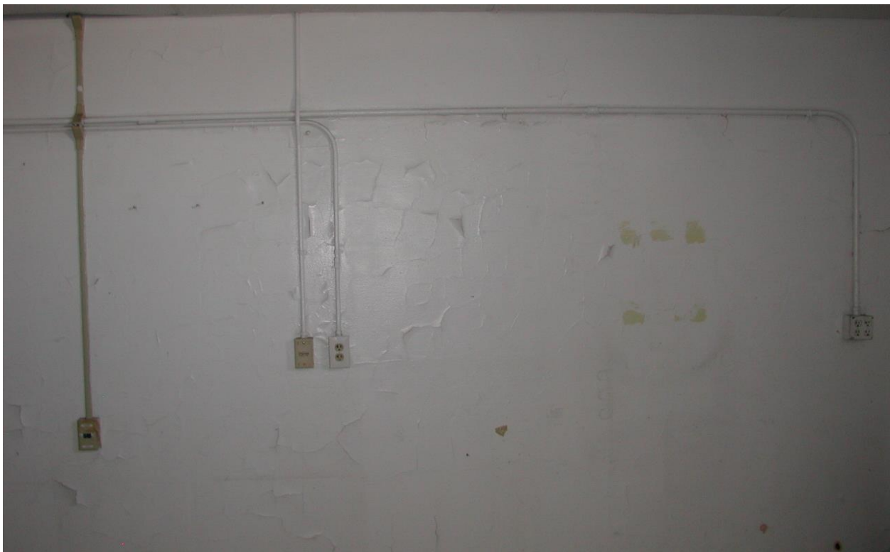
Figure 31. Typical concrete wall in need of repainting (Mr. Richard Simonton, 2013).
