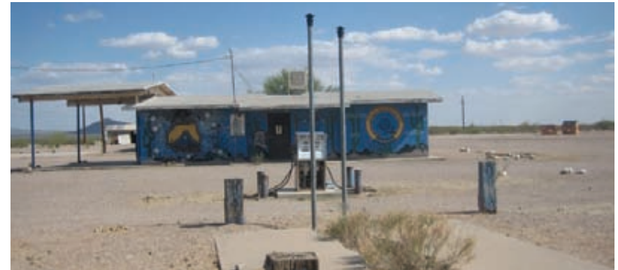
Lower left and above: Cleaning up petroleum contamination at a former Underground Storage Tank site, in Tuba City, Arizona.
