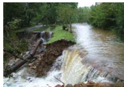
Damage to the city water system in Asheville, North Carolina, due to heavy rain in 2004.
