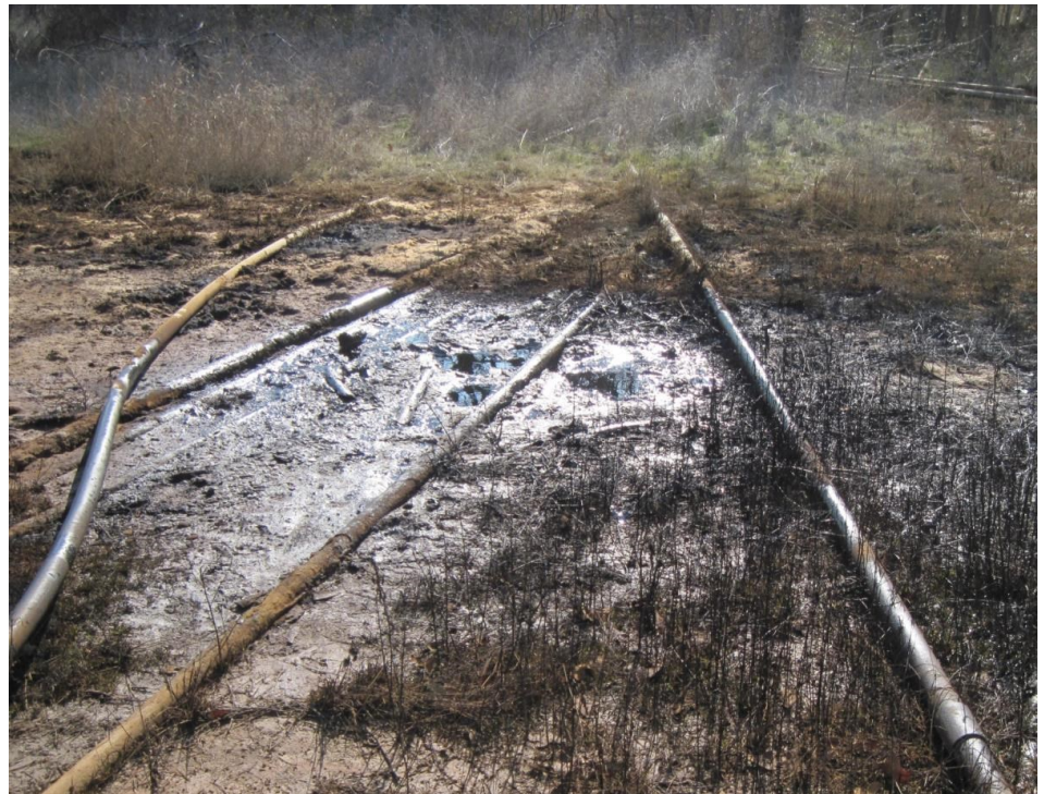
Aging flowlines and corrosion are major cause of oilfield leaks/USFWS
