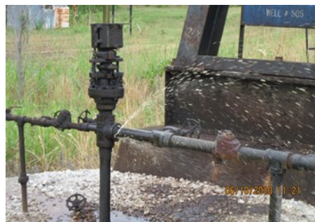
Brine leaking from oil well/USFWS
