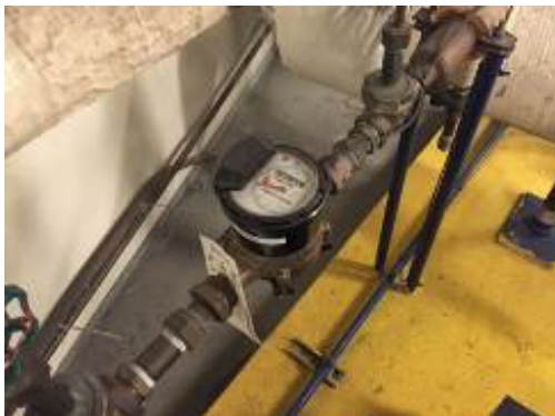
Tracking submeters and utility bills led to finding hidden sources of water waste.
