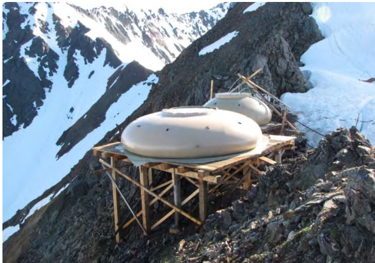
Photo 2-4. Typical water system setup showing collapsible bladders/platform/hose line
