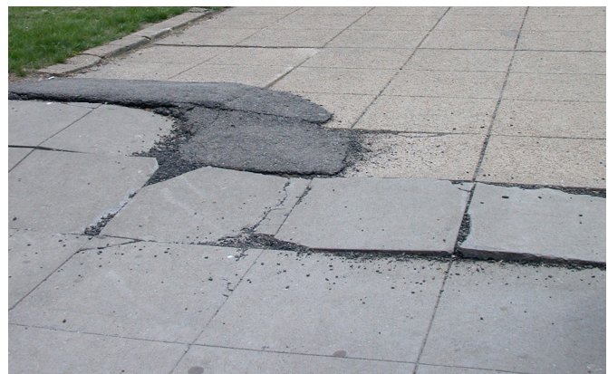
A sidewalk with raised and broken sections is a barrier to access
