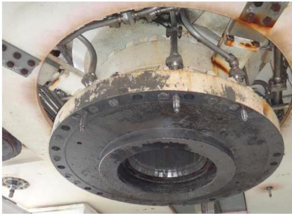
Upper half of failed LMRP Connector
