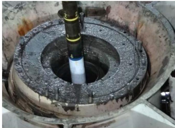
Lower half of failed LMRP Connector
