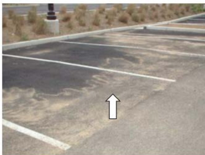
Photo 14-7. Sediment on permeable pavement clogs void spaces thus slowing infiltration. Important to protect permeable pavement from construction stormwater run-off. (Credit: Bill Hunt, NCSU)
