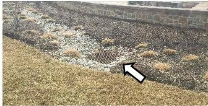
Photo 14-4. If the outlet is set too low, then stormwater will not pond and very little water will infiltrate, as it is designed to do. (Credit: John Kosco, Tetra Tech)
