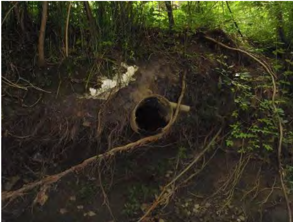
Site: Clyde Paint and Supply Company Site Photograph No.: 8 Direction: NA Subject: Large outfall pipe on east bank of Raccoon Creek
