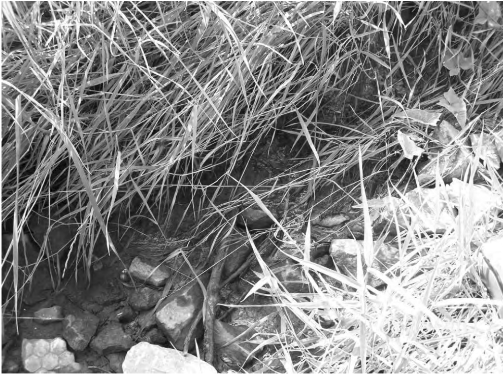
Photo 5: Leachate seep along Raccoon Creek just upstream of “S” curve.
