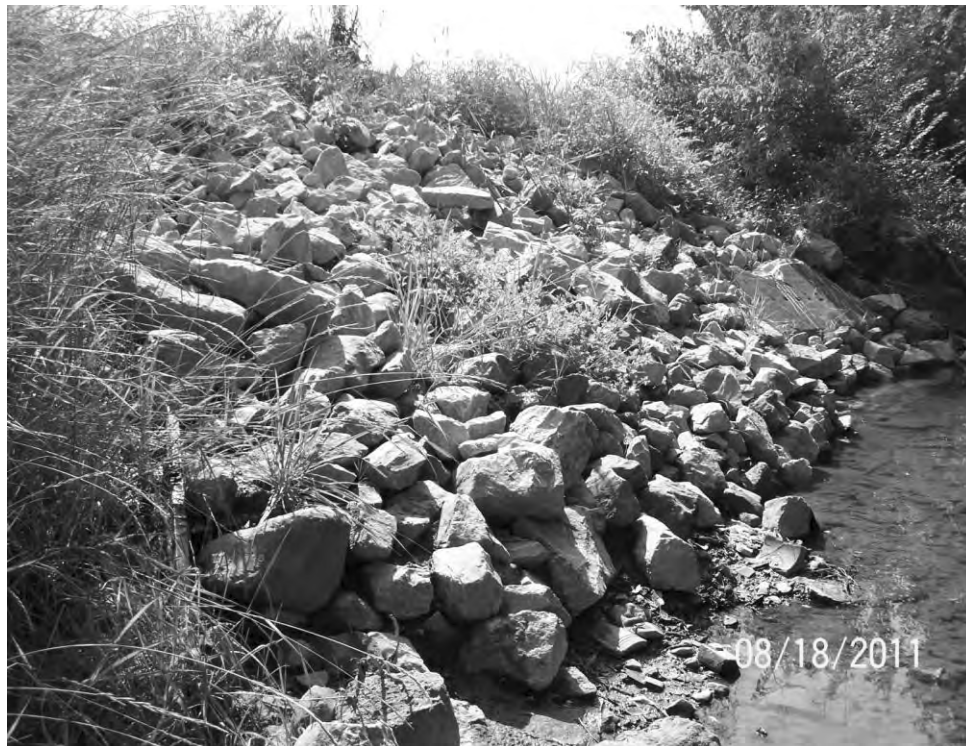
Photo 13: Southernmost riprap area along Raccoon Creek where leachate photos 14 and 15 were taken.
