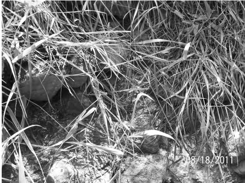
Photo 12: Leachate seep along Raccoon Creek at middle rip-rap area.
