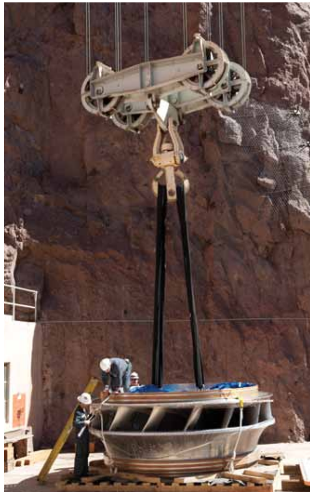
A wide-head turbine – one of the technologies being used to address drought conditions on the Colorado River – is prepared to be transported into the Hoover Dam powerhouse.
