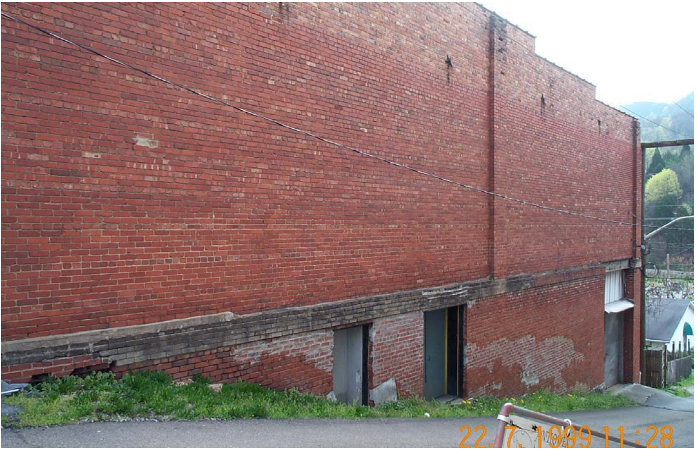
#6 Side View of Karate School, taken from corner of Jackson and Cleveland Streets
