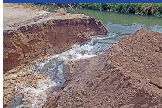
An example of a breach in an earthen canal embankment resulting from rodent activity.
