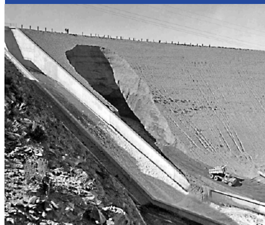
Fontenelle Dam on the Green River in southwestern Wyoming, 1965. Partial failure caused by internal erosion.
