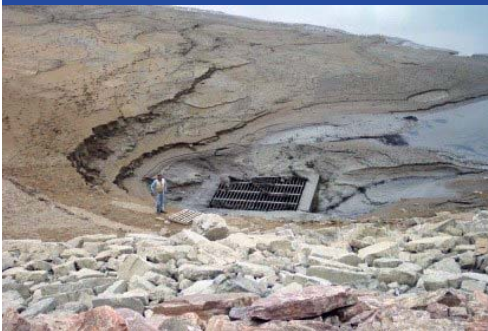
Outlet works impacted by sediment at Belle Fourche Reservoir, South Dakota.
