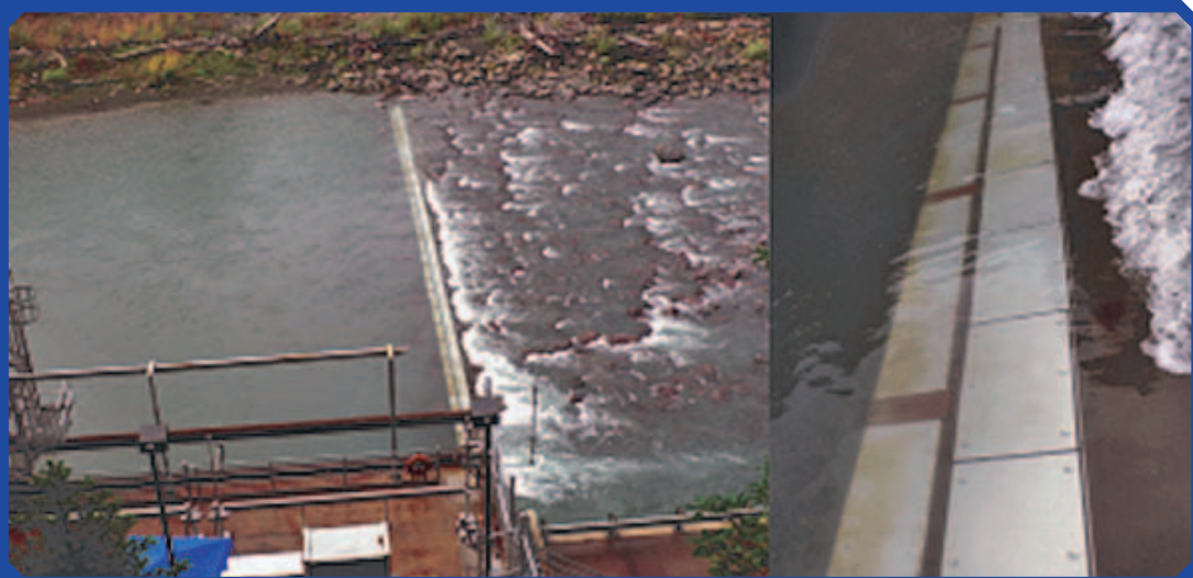
Photograph looking down on the Elwha River impact plate system and surface water diversion structure (left). Closeup photograph of the impact plates mounted on the downstream side of a concrete weir (right). In both images the flow of water is from left to right.
