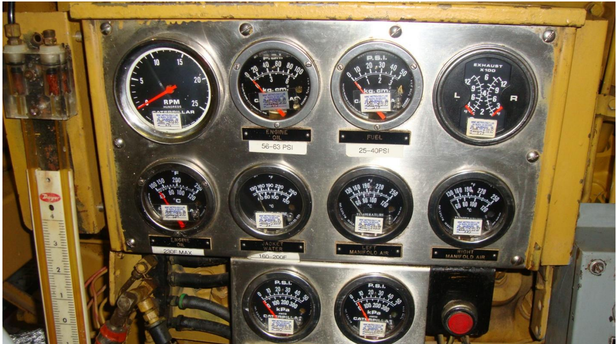
Figure 6. Engine Local Operating Panel
