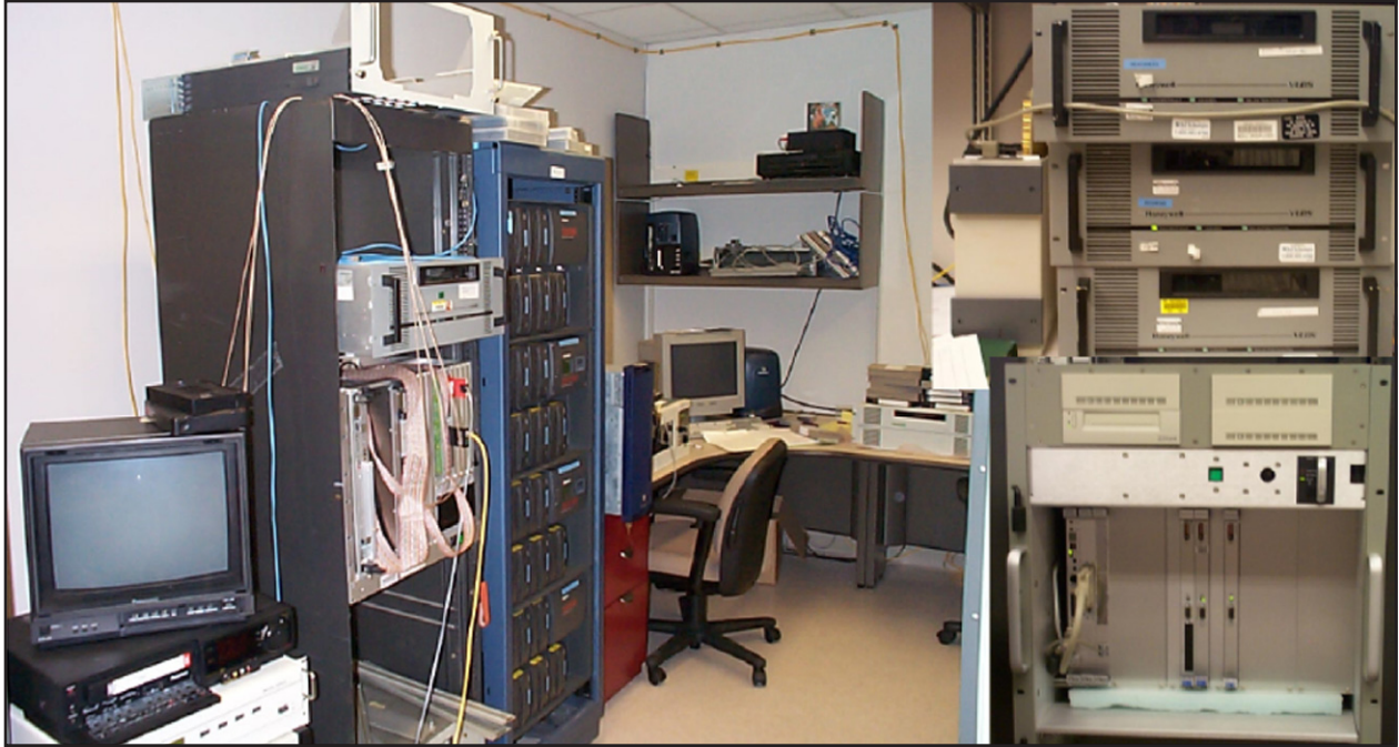
Radar Imaging Facility RAID storage system, real-time processor, and VLDS recorder units
