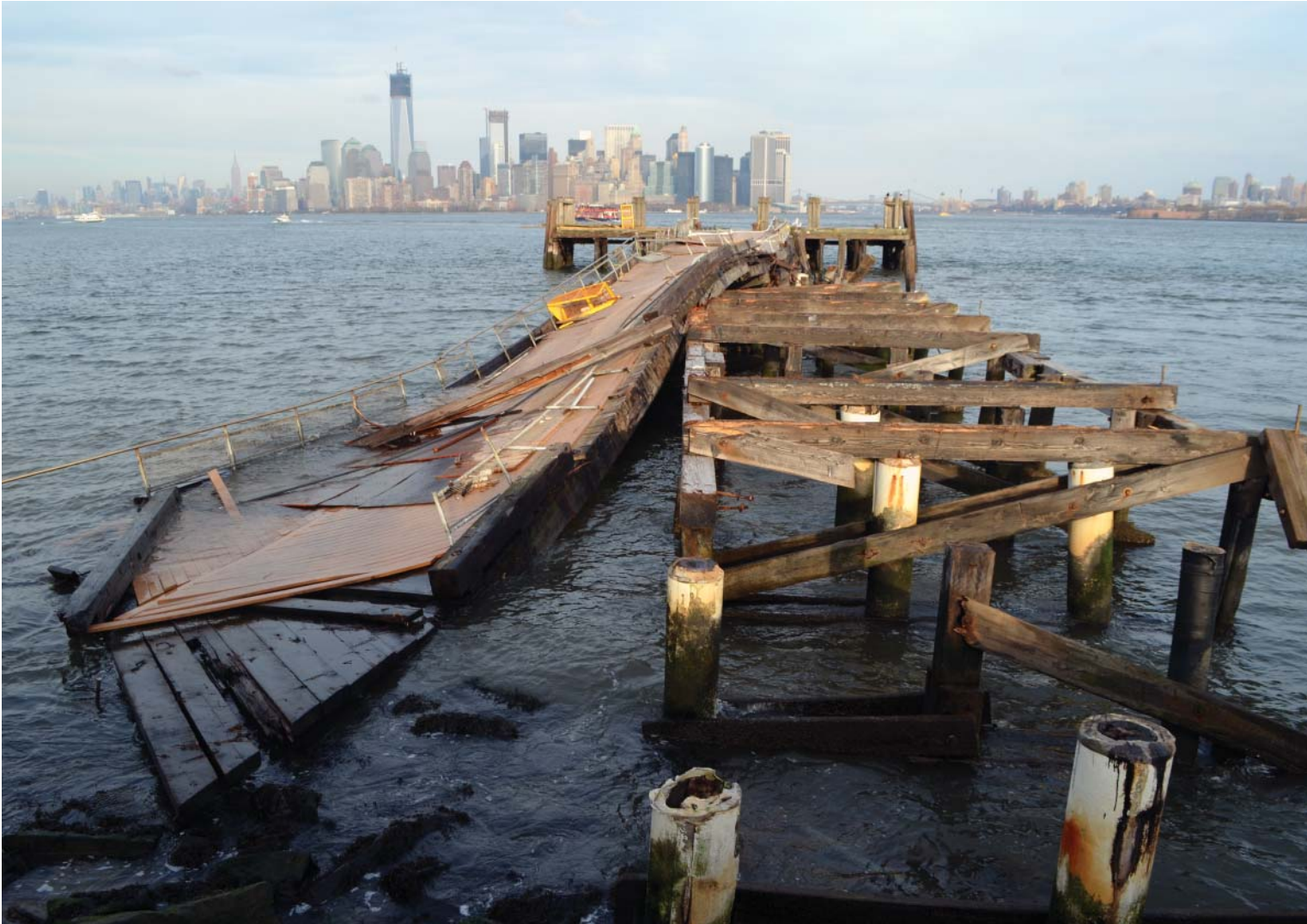
Figure 2. Damaged by Hurricane Sandy in November 2012, this dock at Liberty Island in New York Harbor is a stark reminder of the combined effects of sea-level rise and storm surge. As sea levels increase, severity of potential storm surge also increases. Storm surge is often overlooked by managers planning for the impacts of sea-level rise.
