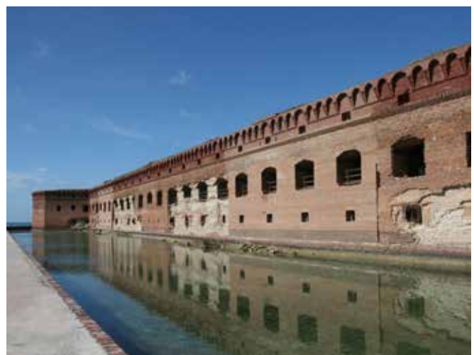
Fort Jefferson needs repairs to its front and moat wall. Image credit: Kelly Clark, NPS.
