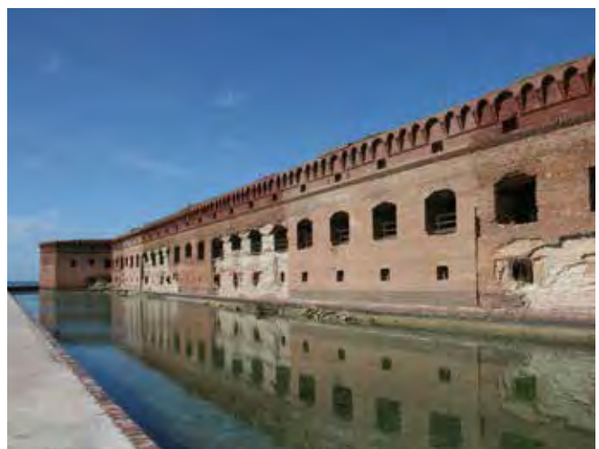
Fort Jefferson needs repairs to its front and moat wall. Image credit: Kelly Clark, NPS.
