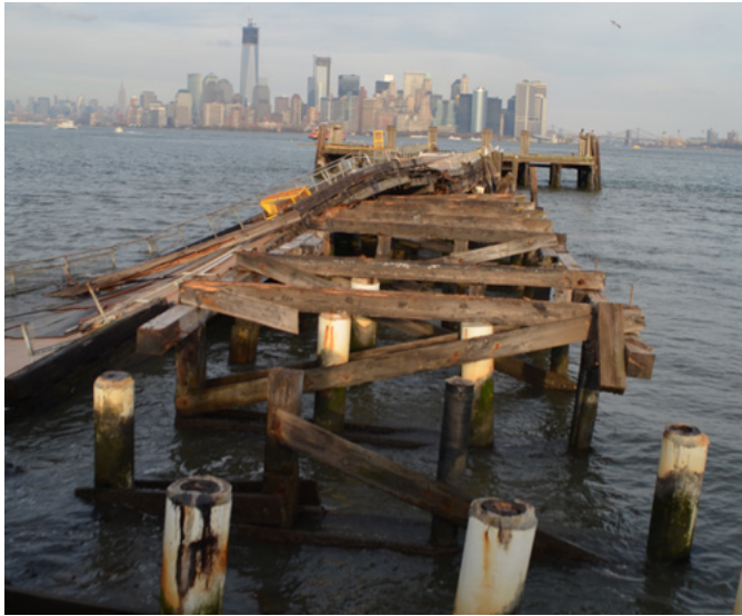
Figure 9.4. Photo from Liberty Island of damaged dock access. Photograph by Rebecca Beavers, NPS.
