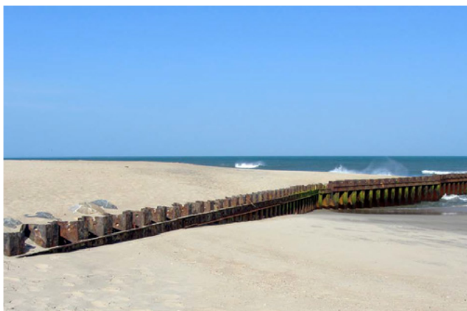
Figure 8.5. Steel sheet-pile groin at the former location of the Cape Hatteras Lighthouse. Photograph by NPS.
