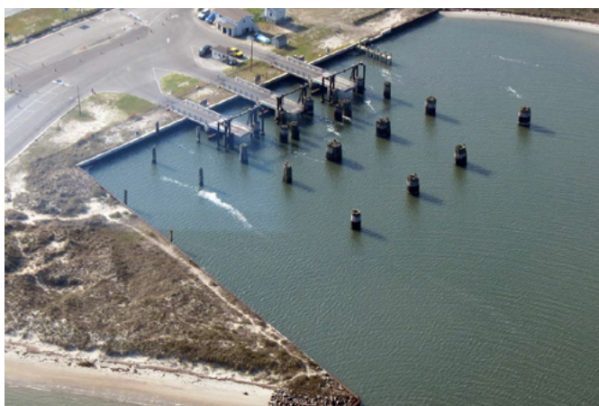
Figure 8.3A. Bulkheads at the Hatteras Island ferry landing on Ocracoke Island, NC. Photograph by NPS.
