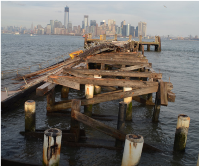
Figure 9.4. Photo from Liberty Island of damaged dock access. Photograph by Rebecca Beavers, NPS.
