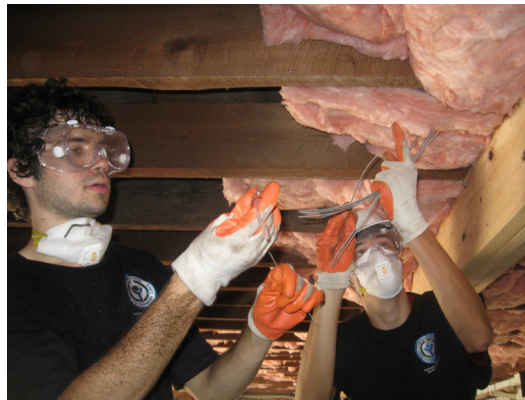
Dennis Walsh and John Mentzer installing insulation in an old barn at Valley Forge NHP that has been retrofitted into a garage and gym.
