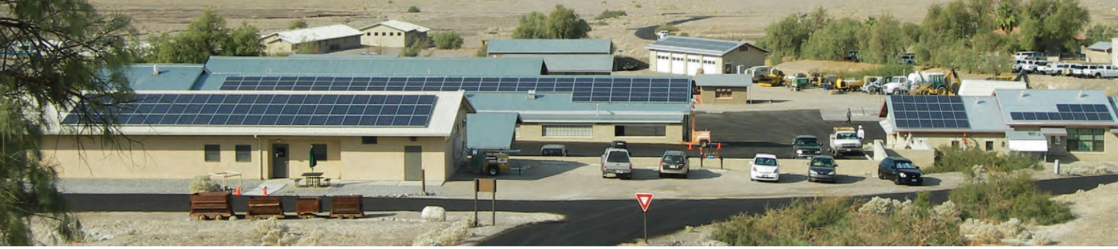
Photovoltaic system, Death Valley National Park, NPS Photo
