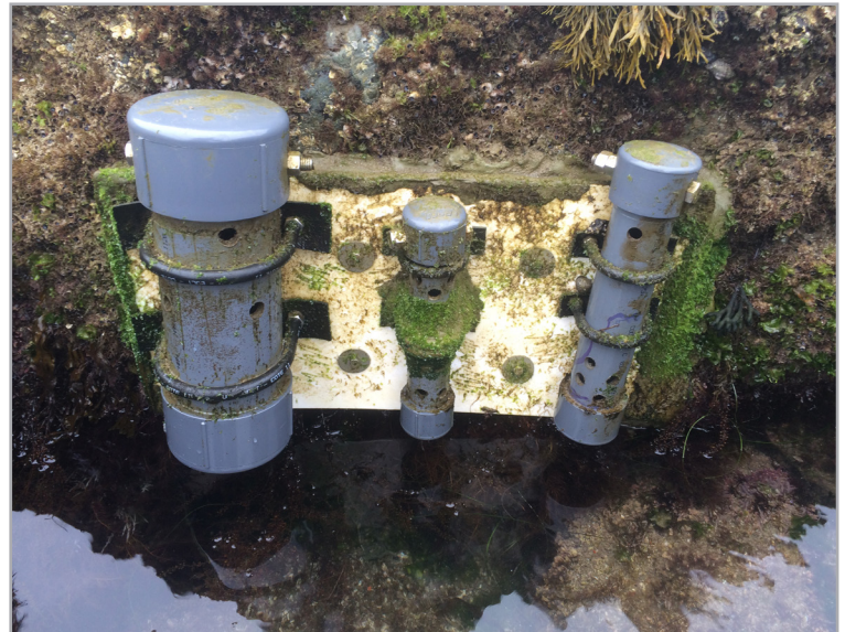
Installation of sea level pressure transducer (left), conductivity sensor (middle), and dissolved oxygen sensor (right) during low tide. Together, these instruments provide additional climate change data that complement the ocean acidification monitoring program. NPS photo by Jonathan Jones
