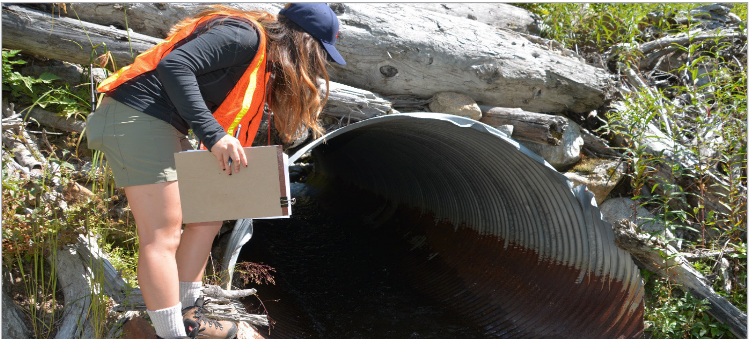
YLCC intern Angelina Ngyuen performs a culvert survey at a road-stream intersection in North Cascades National Park. NPS Image
