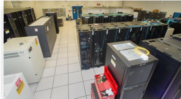
Existing RHIC/ATLAS Computing Facility
