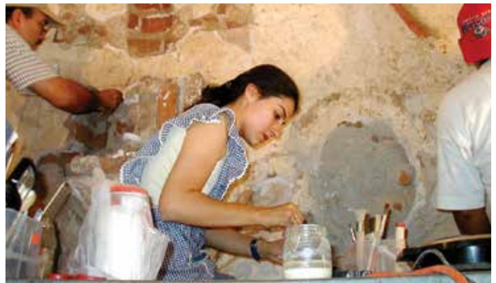
Detailed preservation work on adobe at Tumacácori National Historical Park (NPS photo).
