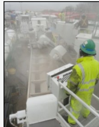
Airborne silica dust at sand mover and transfer system.
