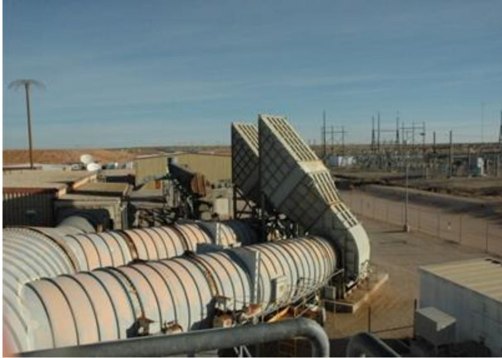
Figure 19: Ventilation Fans 700A and 700B
