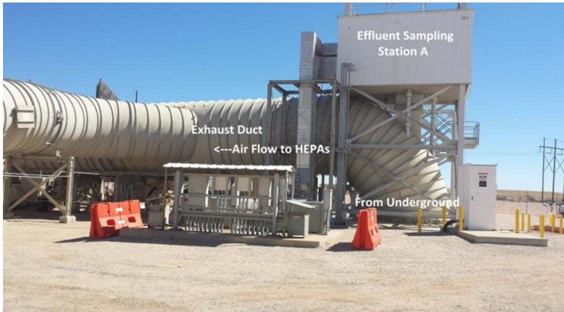
Figure ES-2: Exhaust Air Shaft and Effluent Sample Station A
