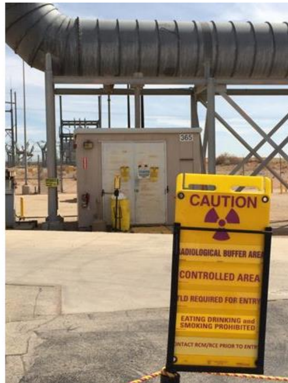
Figure 9: Ventilation Sample Station B
