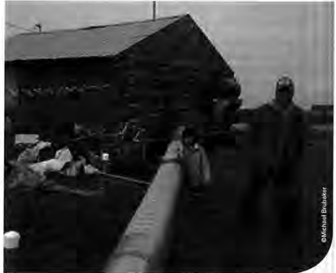
Rising temperatures are causing damage in Native villages in Alaska as sea ice declines and permafrost thaws. Resident of Selawik, Alaska, and his granddaughter survey a water line sinking into the thawing permafrost, August 2011.
