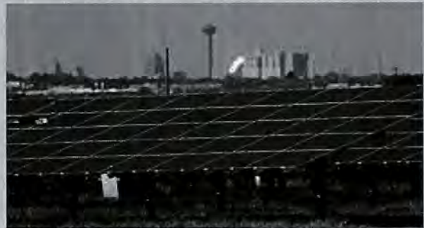
Figure 10.8. Photovoltaic panels convert sunlight directly into electricity. Utility-sized solar power plants require large tracts of land. Photo shows Duke Energy's 113-acre Blue Wing Solar Project in San Antonio, Texas, one of the largest photovoltaic solar farms in the country. (Photo credit: Duke Energy 2010 36 ).
