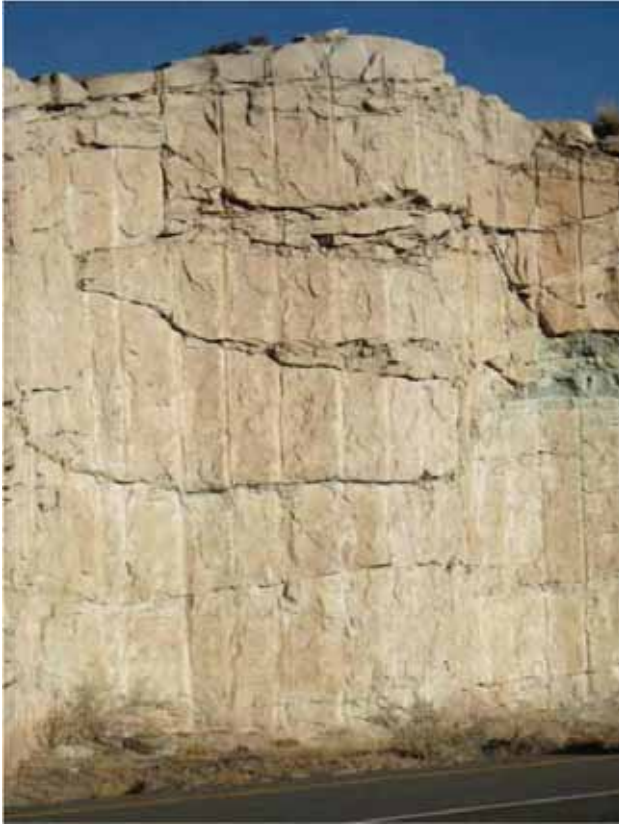
Half cast drill traces in sandstone have an obvious artificial appearance. (Credit: U.S. Department of Transportation Federal Highway Administration.)
