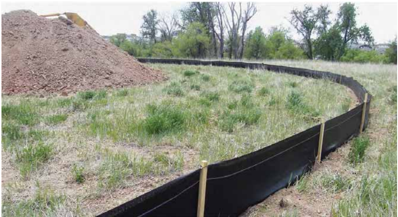
Stockpiled topsoil, surrounded by a silt fence intended to control offsite soil transport during heavy rains. (Credit: BLM.)
