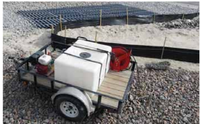
An exit tire wash removes dust, soil, mud, and other materials from trucks to minimize potential trackout of material onto roadways. (Credit: Tom Gore, Altitude Training.)
