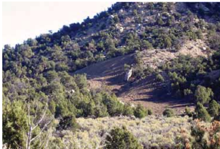
Burying a pipeline. Slopes are contoured to approximate naturally occurring slopes. (Credit: Rob Sweeten, BLM.)
