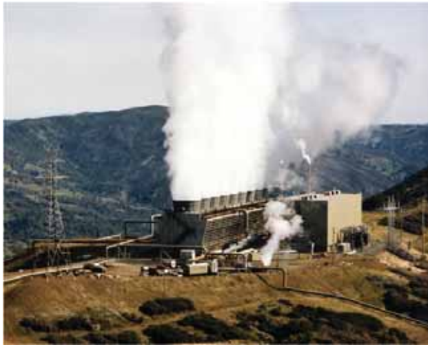
Steam plumes rise from cooling towers at a dry steam plant. (Geysers facility near Calistoga, California. Credit: NREL.)
