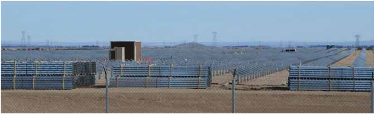
A clean and orderly worksite has fewer negative visual impacts and promotes a positive image of the developer and the BLM. (Credit: Robert Sullivan, Argonne National Laboratory.)
