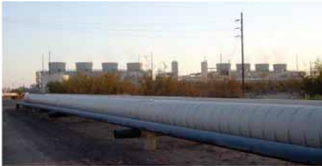
Pipelines and cooling towers at operating geothermal plant. (GEM 2/GEM 3 facility near Holtville, California. Credit: Robert Sullivan, Argonne National Laboratory.)
