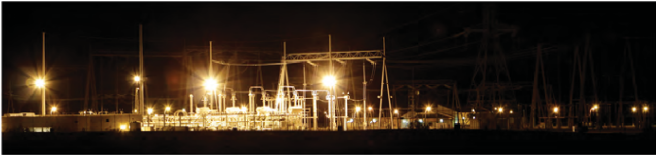
Nighttime shot of a large substation. Numerous bright, poorly shielded lights make this facility a strong source of glare and light spill. (Eldorado Valley, near Boulder City, Nevada. Credit: Marc Sanchez, BLM.)
