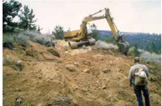
Slope recontouring to approximate naturally occurring slopes during road reclamation. (Credit: BLM.)
