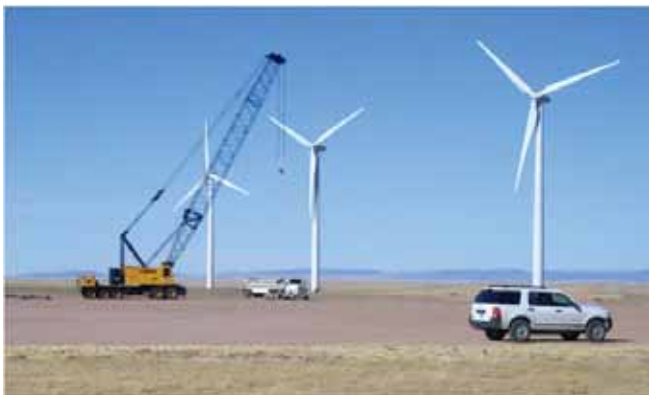
Wind turbine maintenance. (Dunlap Ranch Wind Energy Project near Medicine Bow, Wyoming. Credit: Robert Sullivan, Argonne National Laboratory.)
