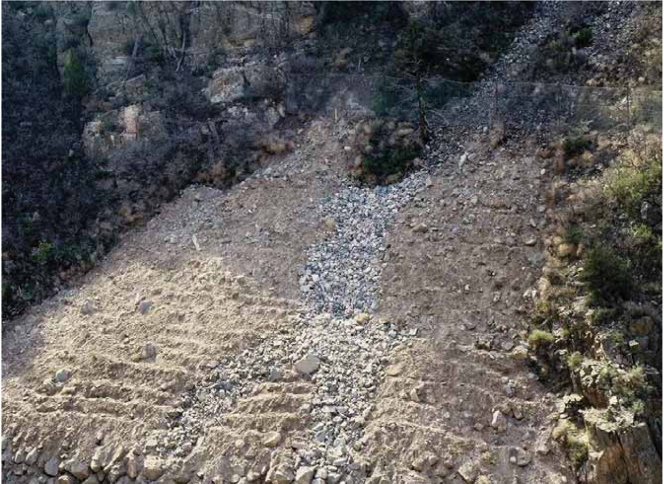
Furrowing slopes results in increased water retention, reduced erosion, and better revegetation. (Credit: John McCarty, Colorado Department of Transportation.)
