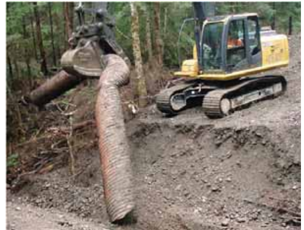
Culvert removal during road decommissioning. (Credit: Washington State Recreation and Conservation Office.)
