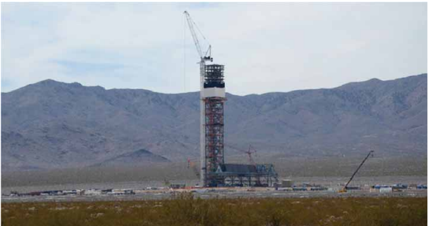
Ivanpah Solar Energy Generating System power tower under construction. The grayish area at center is a heliostat field for the central tower, one of three towers in the facility. The structure just to the right of the tower base will house the steam turbine generator. (Credit: Robert Sullivan, Argonne National Laboratory.)
