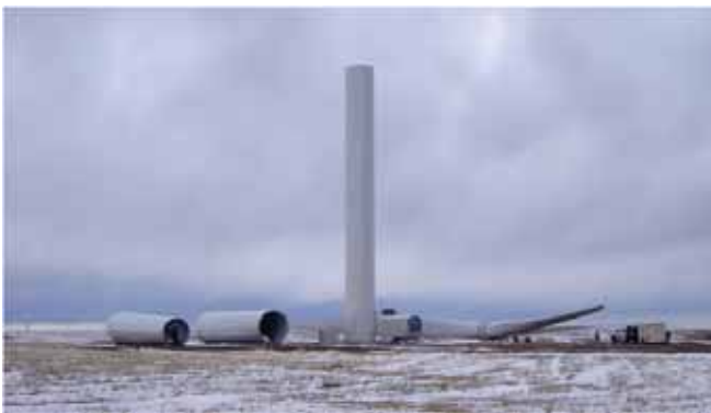
Partially erected turbine, with nacelle and hub visible at right center. (Near Peetz, Colorado. Credit: Robert Sullivan, Argonne National Laboratory.)
