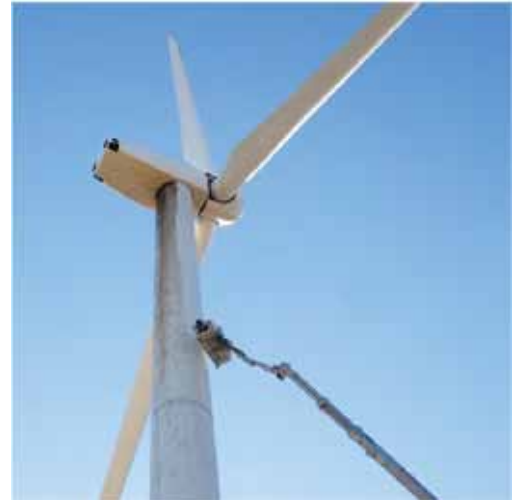
Cleaning leaking fluid from a wind turbine. (Credit: TGM Wind Services)
