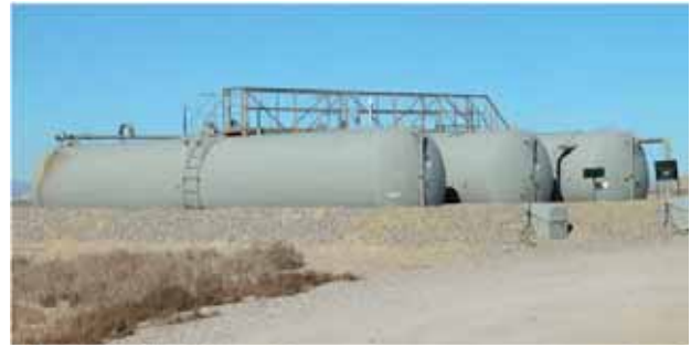
Horizontal tanks reduce tank height substantially. (Credit: John McCarty, BLM.)
