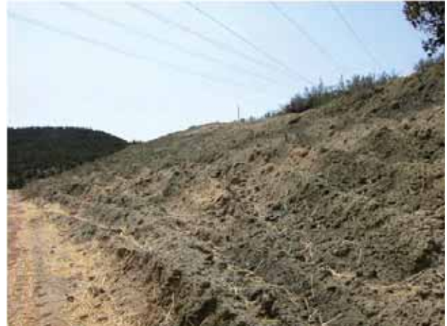
This roughened slope will revegetate faster and more completely than a smooth slope. (Credit: BLM.)
