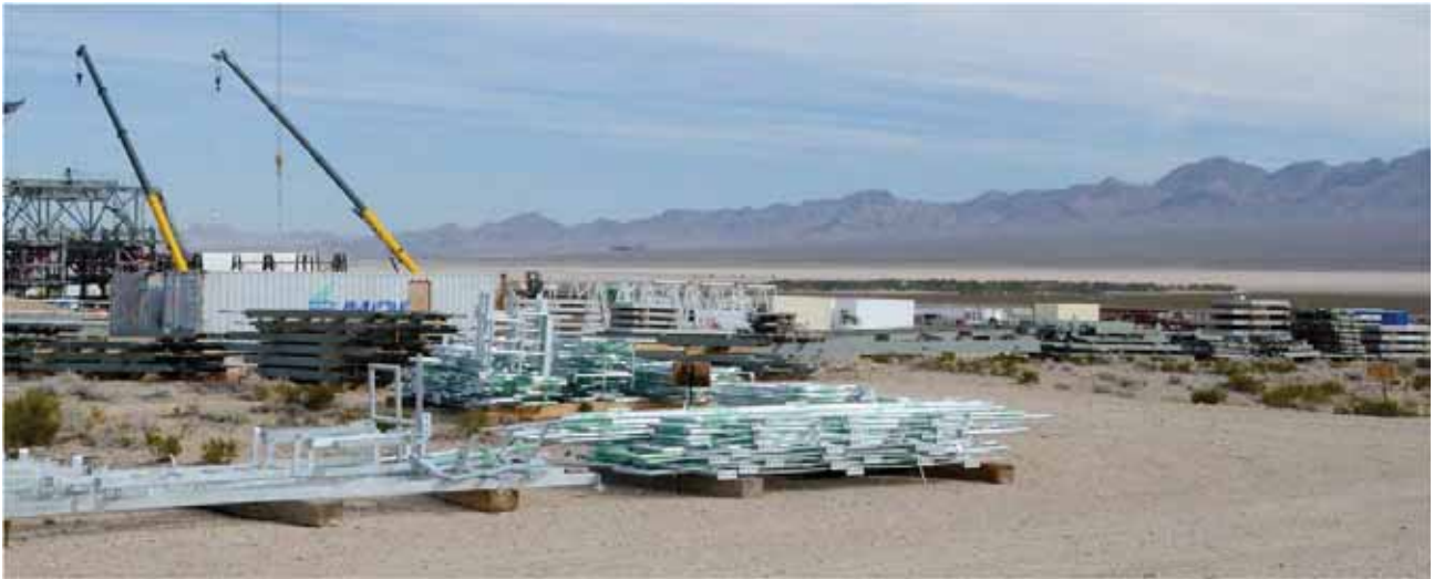
Staging area at Ivanpah Solar Energy Generating System power tower facility, Ivanpah Valley, California. (Credit: Robert Sullivan, Argonne National Laboratory.)
