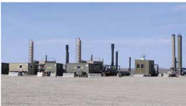
These grouped structures have been painted a variety of colors that do not match each other. (Credit: BLM.)
