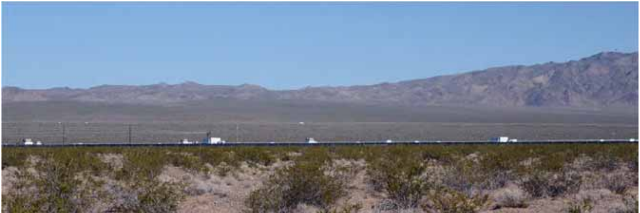
White power conversion units (inverters) at thin-film PV facility contrast strongly with vegetative backdrop. (Credit: Robert Sullivan, Argonne National Laboratory.)
