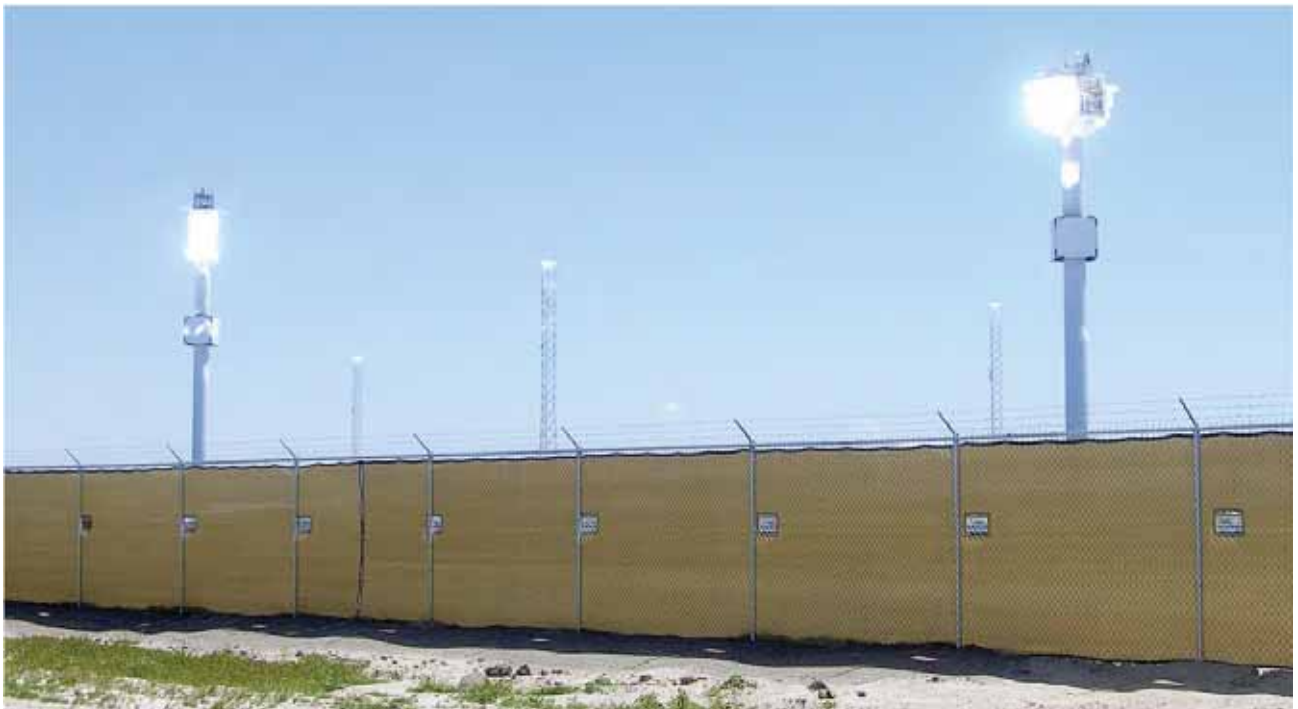
A fabric-covered screening fence at power tower facility screens the heliostats, but not the receivers. (eSolar Sierra Suntower, Lancaster, California. Credit: Robert Sullivan, Argonne National Laboratory.)
