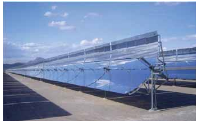
Parabolic trough assembly at a parabolic trough facility, including large curved reflectors, the HTF tube at the focal point of the reflectors, and the support structure behind and below the reflectors. (Nevada Solar One near Boulder City, Nevada. Credit: Robert Sullivan, Argonne National Laboratory.)
