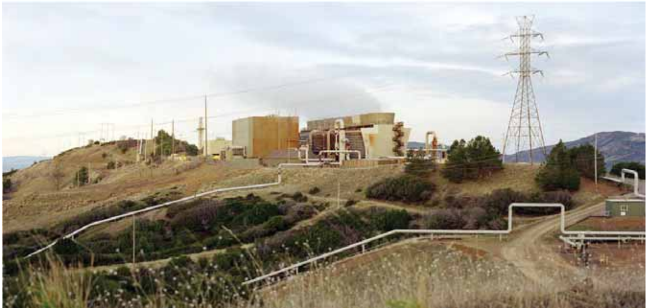
Uncoated geothermal pipelines contrast strongly with their surroundings. (Geysers facility near Calistoga, California. Credit: David Parsons, NREL.)
