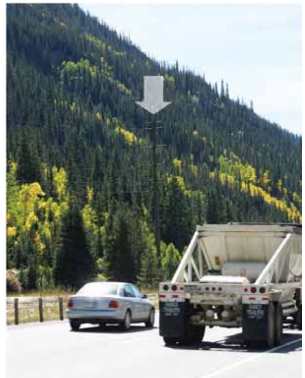
This color-treated monopole transmission tower repeats the line and color of the surrounding vegetation effectively, even at a short viewing distance. Only the horizontal line contrast from reflections of sunlight on the upper sides of the crossbars stands out from the background. (Credit: John McCarty, BLM.)
