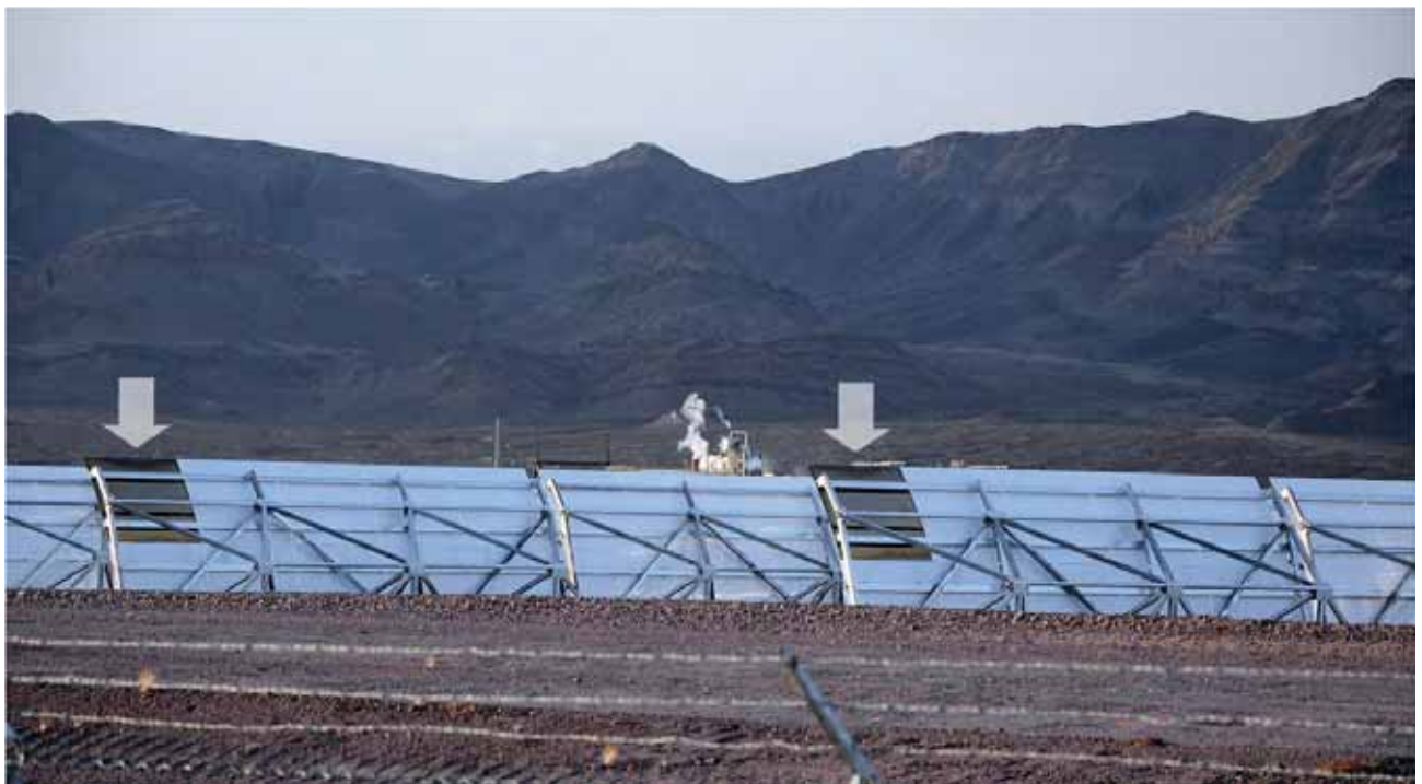
Close-up view of experimental application of color-treated trough mirror backs (visible at left and center) at a parabolic trough facility. Untreated mirror backs appear blue. (Nevada Solar One facility near Boulder City, Nevada. Credit: Robert Sullivan, Argonne National Laboratory.)
