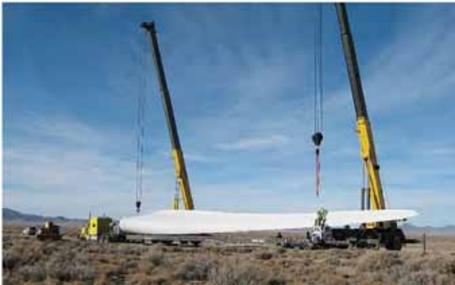
Unloading a wind turbine blade. (Milford Wind Corridor project, near Milford, Utah. Credit: BLM.)
