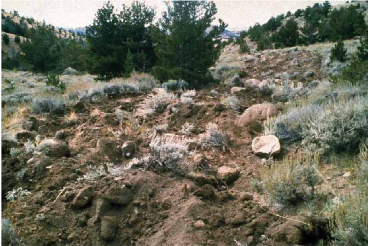
Road removal in progress. The flat road surface is roughened, rocks are added, and vegetation transplanted from the edges of the ROW. (Credit: BLM.)
