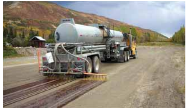
Application of dust palliative. (Credit: Alaska Department of Environmental Conservation, Division of Air Quality.)
