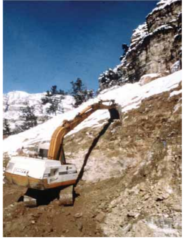
Proper replacement of this rock shelf preserves the form, line, and texture of the original rock shelf, and color contrast will be greatly reduced when revegetation occurs. (Credit: John McCarty, Colorado Department of Transportation.)
