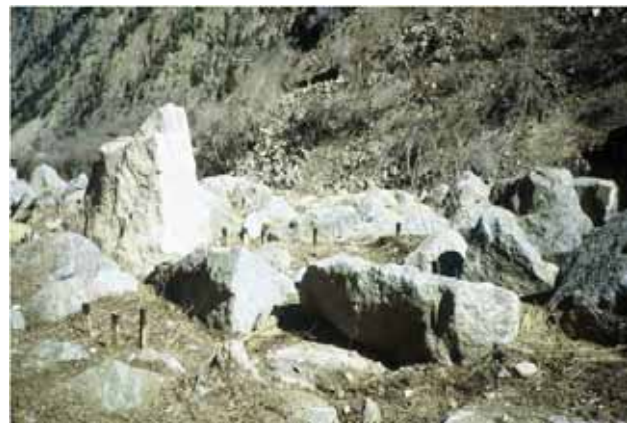
The placement of salvaged rocks on this slope helps to restore a more natural appearance to the reclaimed area, and holds soil in place for successful revegetation. (Credit: John McCarty, Colorado Department of Transportation.)
