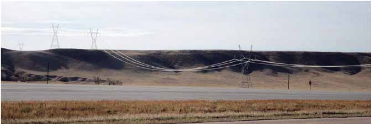
Failure to employ non-specular conductors for this transmission line result in high visual contrast in sunny conditions. (Credit: Robert Sullivan, Argonne National Laboratory.)
