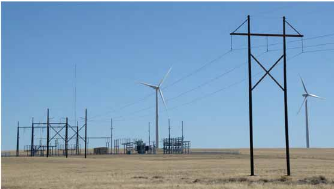
Wind energy facility substation, with meteorological tower in background. (Dunlap Ranch Wind Energy Project near Medicine Bow, Wyoming. Credit: Robert Sullivan, Argonne National Laboratory.)
