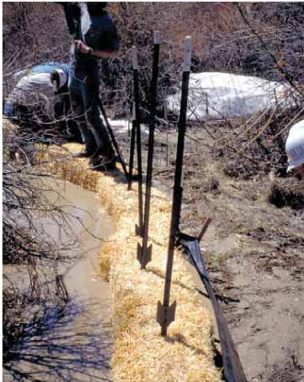
Although imperfectly installed, this combination of straw bales and silt fence is holding back a large amount of water and sediment. (Credit: John McCarty, BLM.)
