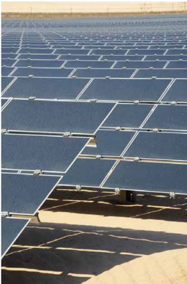
Flat plate PV: Thin-film PV panels on fixed (non-tracking) mounts. (Silver State North Solar Project near Primm, Nevada. Credit: Robert Sullivan, Argonne National Laboratory.)
