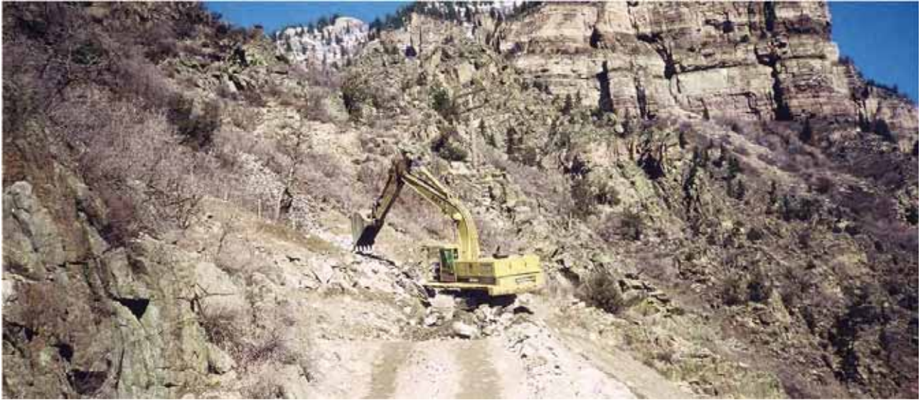
Slope recontouring for road reclamation. (Credit: John McCarty, Colorado Department of Transportation.)
