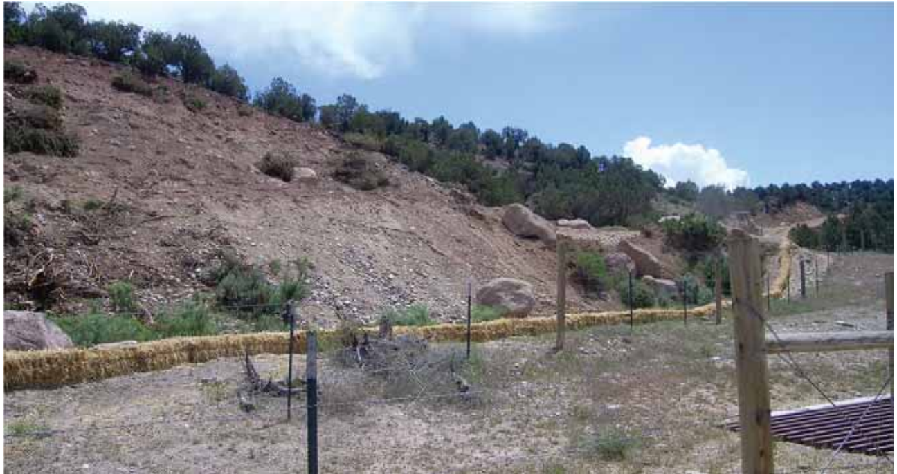
An example of erosion control good practices: straw bales used for downslope sediment control. (Credit: BLM.)
