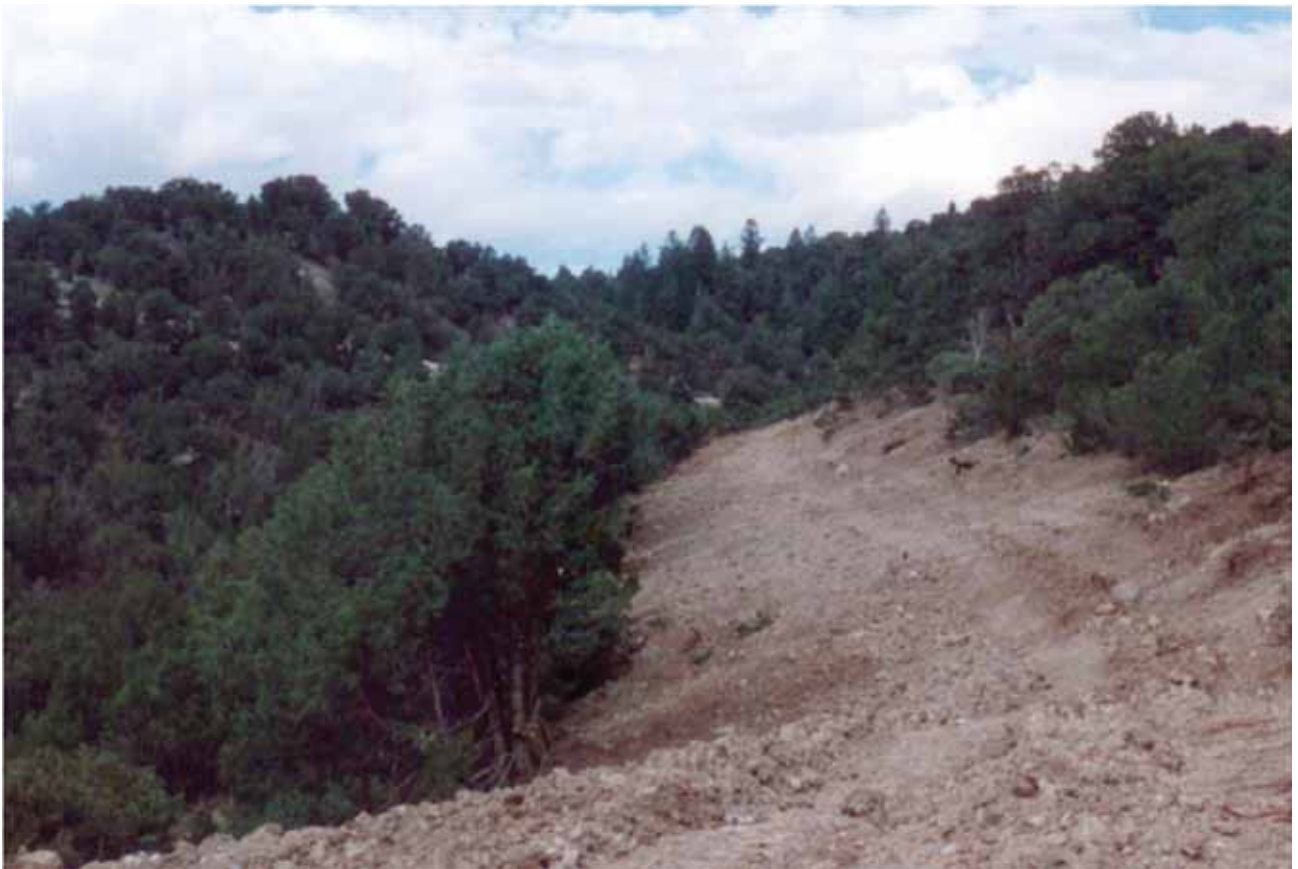
The recontoured slope for this reclaimed road blends in well with the naturally occurring slope. (Credit: BLM.)
