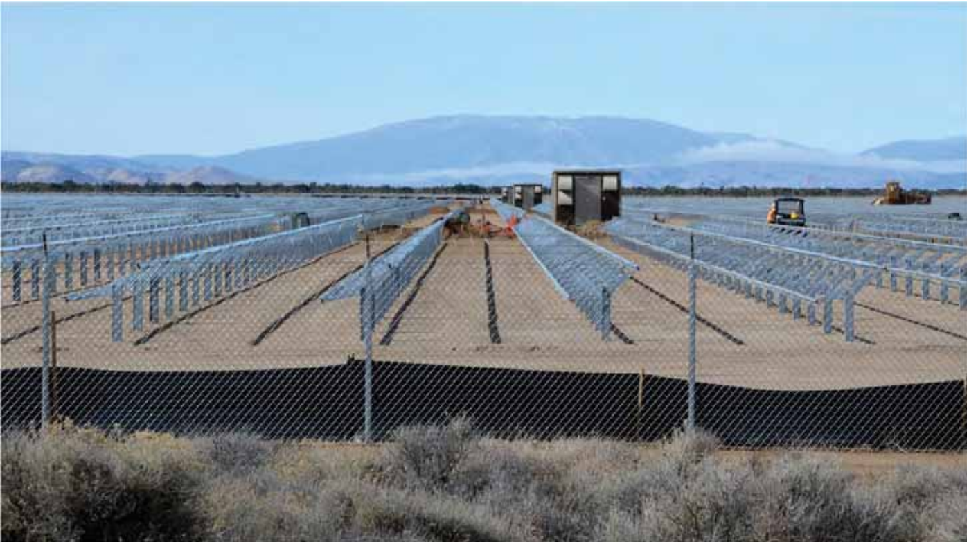
Antelope Valley Solar Ranch thin-film PV facility under construction. Fixed (non-tracking) mounts for the PV panels have been installed, and await the panels. Note complete clearing of vegetation and leveling of ground underneath the collectors. (Credit: Robert Sullivan, Argonne National Laboratory.)
