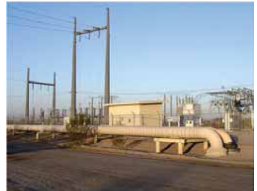
Geothermal pipelines coated to match surroundings at dual-flash geothermal power plant. Note that better results would have been obtained by using a darker color shade on the pipe coating. (GEM 2/GEM 3 facility near Holtville, California. Credit: Robert Sullivan, Argonne National Laboratory.)
