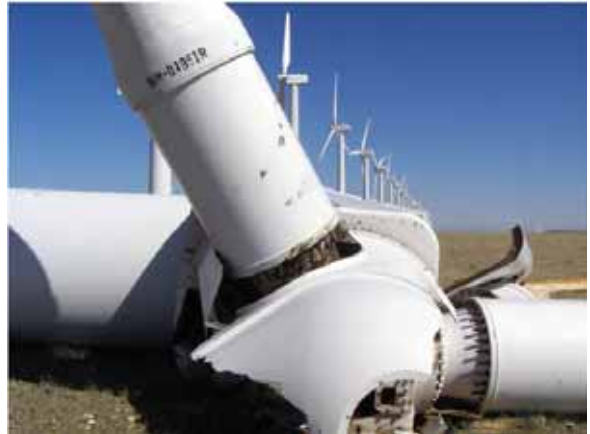
Collapsed wind turbine. (Arlington Wind Farm, Wyoming. Credit: BLM.)
