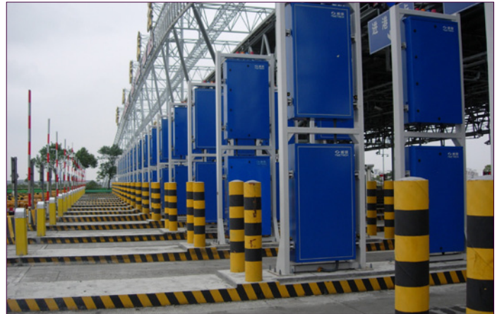
The 17 radiation portal monitors installed at the Port of Yangshan will scan 100% of export containers.
