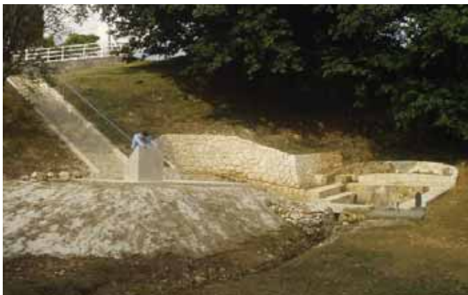
Wide view of the restoration project, showing the new stairway leading to the spring.
