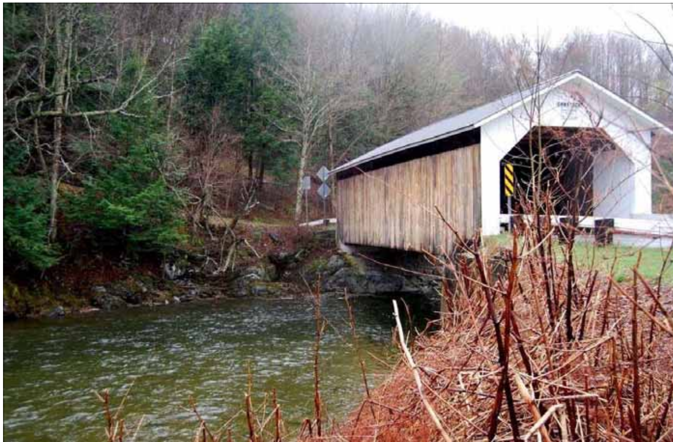
Figure 53. Comstock Bridge, over the Trout River in Montgomery. Photo by Ken Secor
