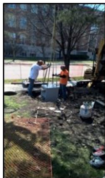
4160V Switch Installed in 2015
