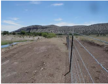
Newly constructed fence excludes livestock from the Rio Penasco and adjacent riparian areas. The river provides recreational trout fishing in this stretch. Photo: USFWS
