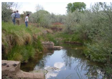
Bank undercutting and slumping prior to Partners project construction near Santa Fe, New Mexico.
